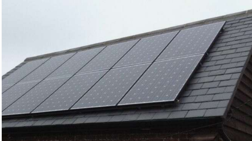
Example of a similar solar panel installation on a slate roof
