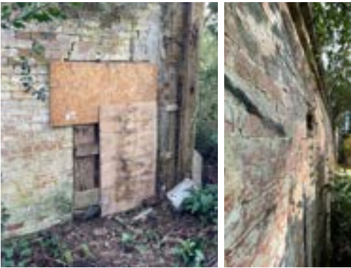
3 - The eastern boundary wall is derelict, with cracks throughout the structure and a high level of damage from climbing plants.
