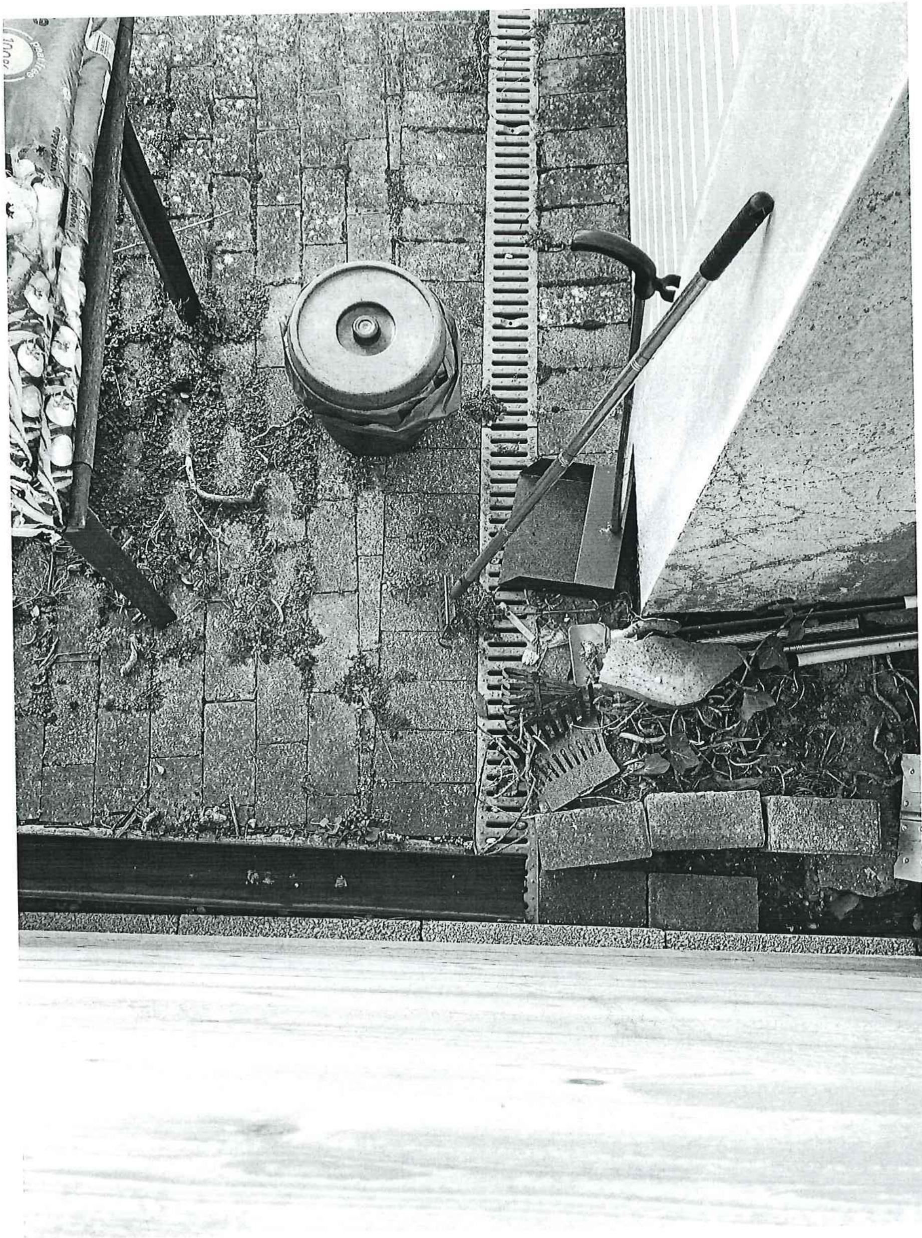
NEW FENCE BASE AND NEW FENCING IN PLACE BUT DRAINAGE FROM 38 YARDLEY ROAD CONTINUES TO FLOW THROUGH INTO MY PROPERTY
