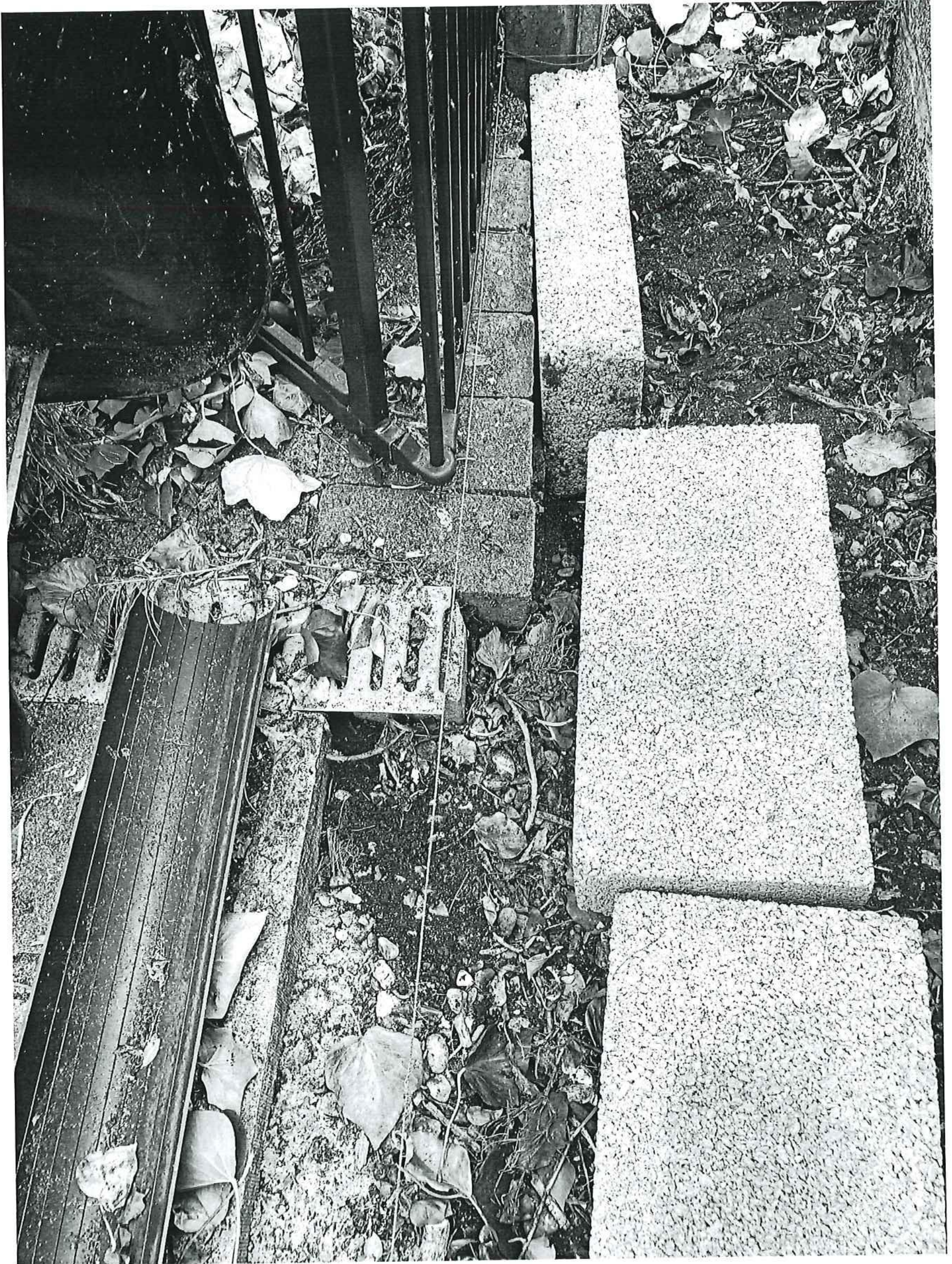
OUTFLOW OF DRAINAGE FROM SOUTH FACING ROOF AND GUTTERING AND DRAINAGE FROM NEW PORCH AND HARD SURFACE DRIVEWAY FLOWS INTO MY PROPERTY HERE . DESPITE FOUNDATIONS FOR NEW FENCING GOING IN THE DRAINAGE FROM NEXT DOOR CONTINUES .
