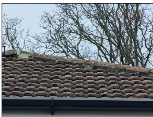
Figure 5 – lifted roof tiles on western roof face
