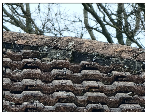
Figure 6 – lifted roof tiles
