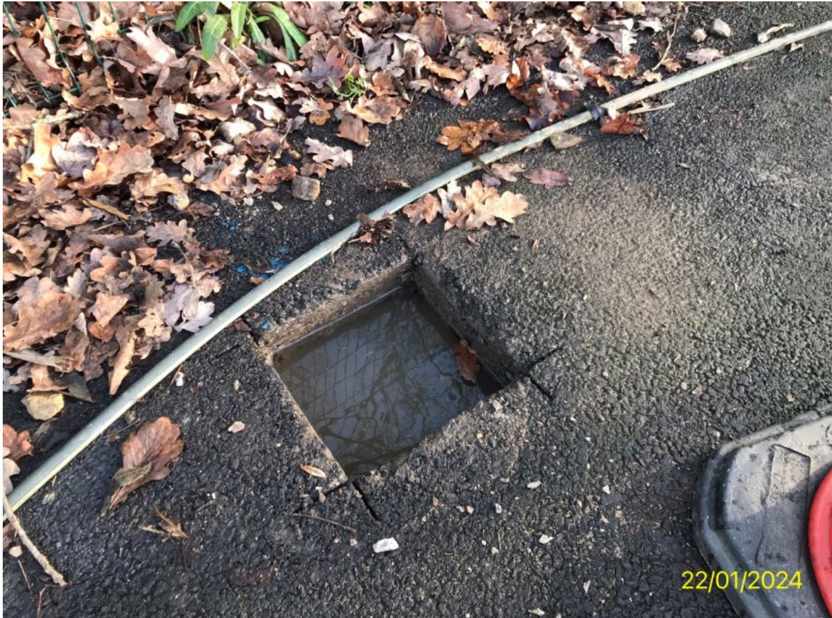
Image 4: Trial Hole 3 tarmac layer, but and below this not visible in this photo because of the water.
