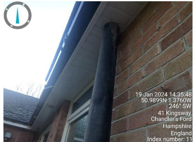
Photograph 14: View of the soffits, which do not provide any gaps for bat access.
