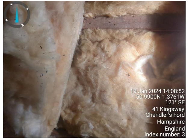
Photograph 26: View of the scattered bat droppings on the insulation.
