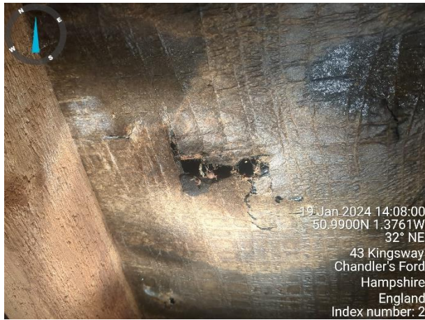
Photograph 25: View of a tear in the bitumen felt lining.
