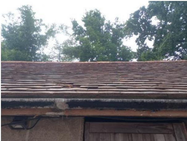
Photo 9: Potential roost feature on garage – damaged/lifted tiles
