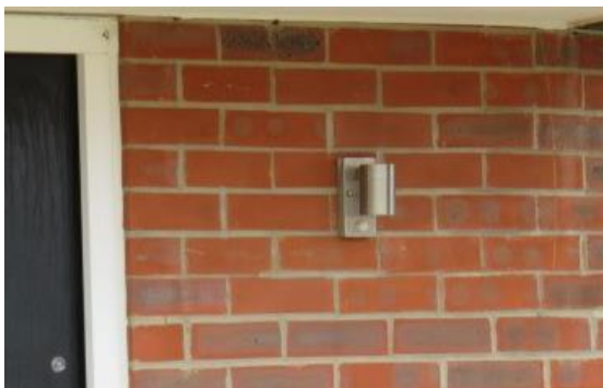
Image showing external lighting in-situ.
