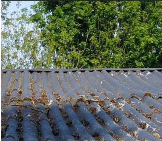
Figure 13. View of gaps underneath metal ridge.
