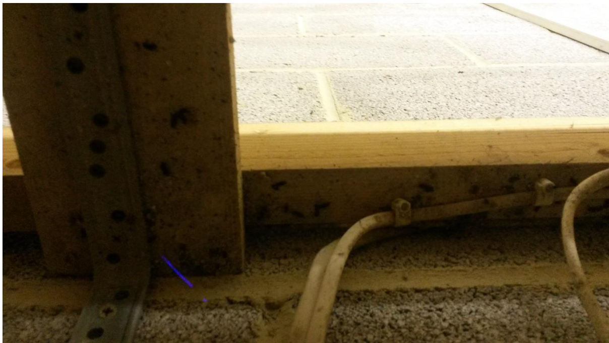
Photo 4: Brown long-eared droppings on beam in attic
