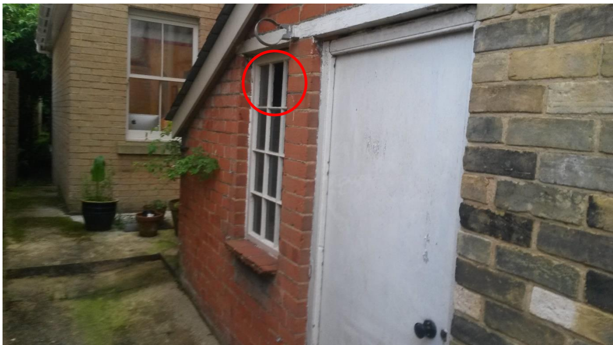
Photo 8: Broken window leading to the cellar/boiler room
