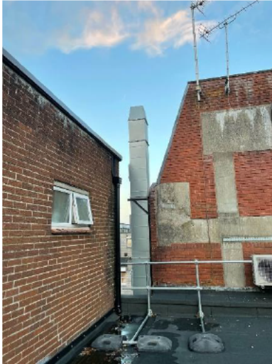
Figure 6.1 – Kitchen Extraction System
