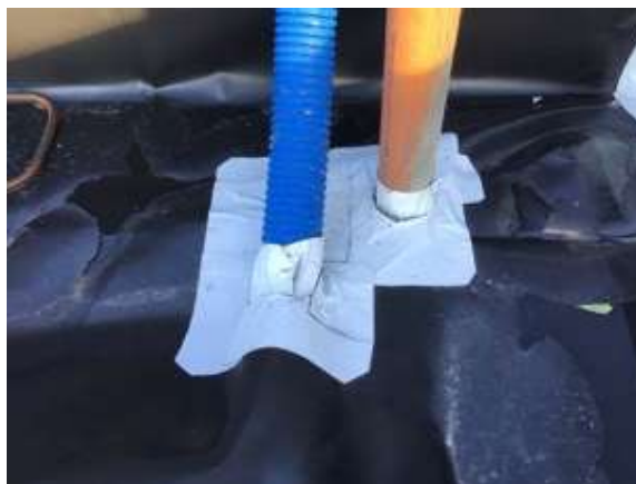
Sealed double pipe penetration using SAGM.
