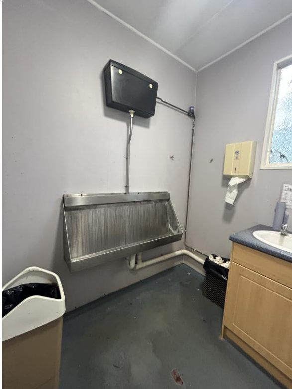
Typical example of sanitary fitting
