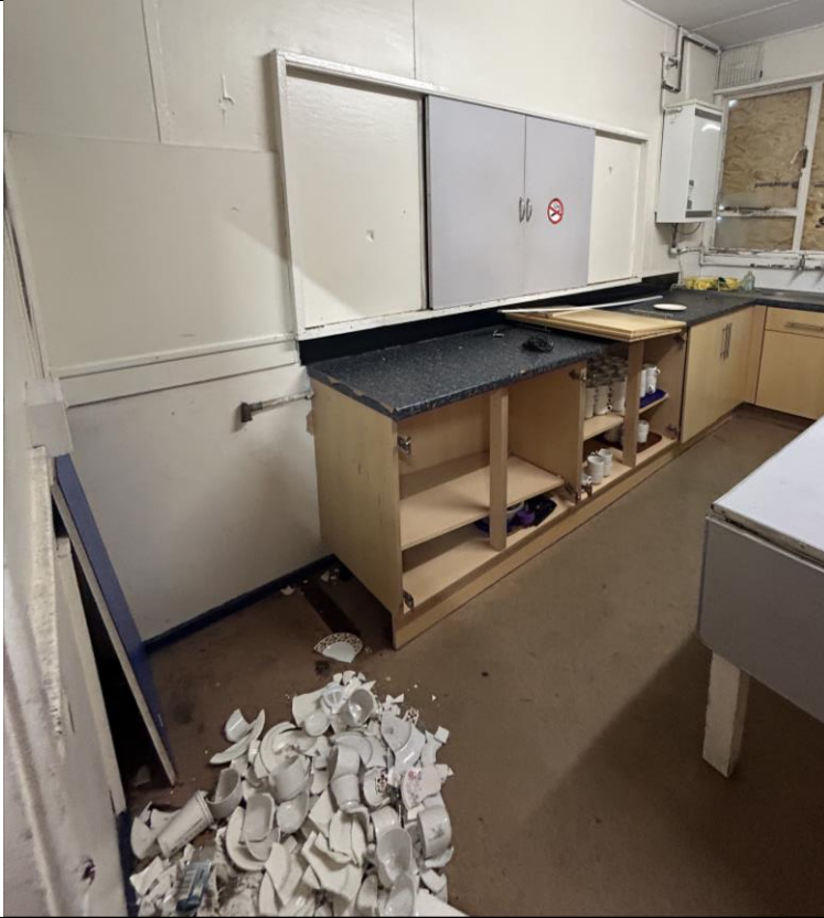
Service hatch between kitchen and hall non-fire rated.
