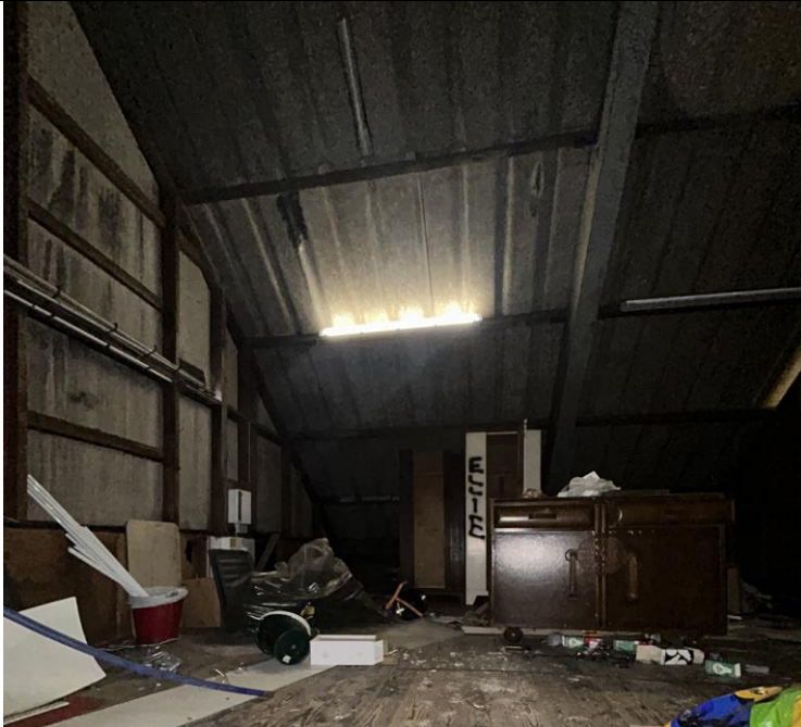
Mezzanine areas water staining to back of AC roof sheets.
