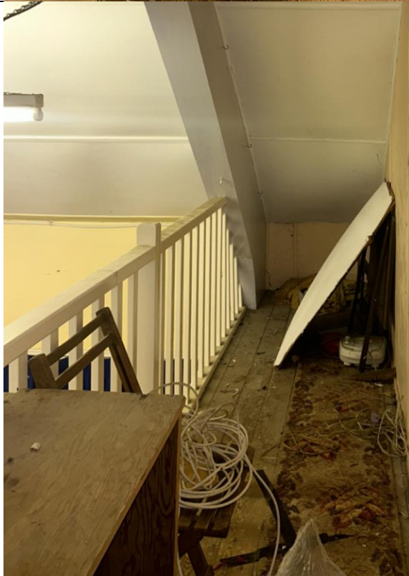
Mezzanine balcony handrail below current standards.
