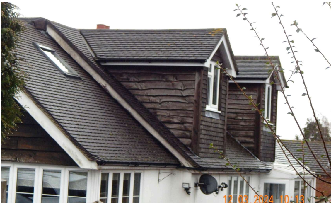
Image 2 – South facing elevation of the property offering vertical timber claddings to the former windows where gaps of adequate proportions to offer likely shelter for crevice dwelling bats were observed
