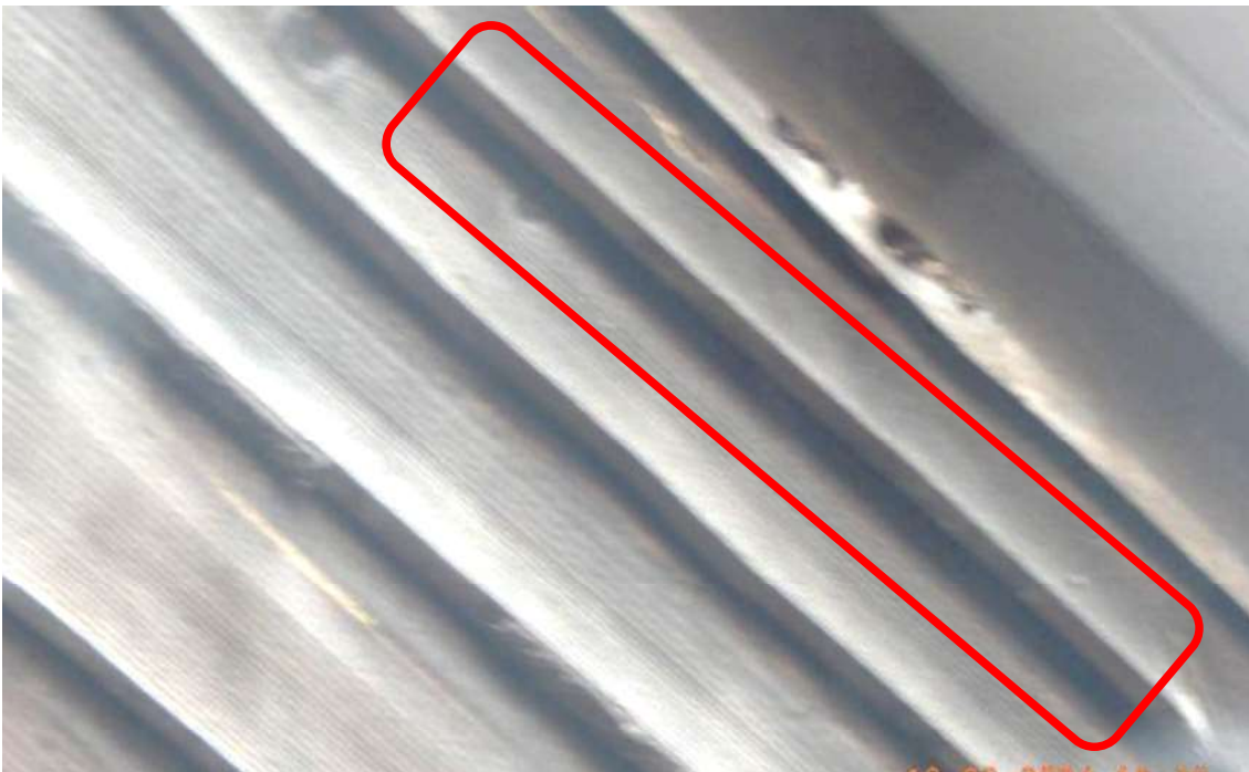
Image 4 – Example of gaps within the timber claddings as per images two and three
