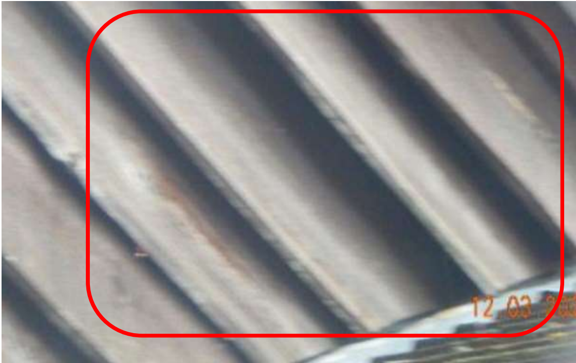
Image 5 – Example of gaps within the timber claddings as per images two and three
