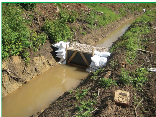
Figure 4.57 Silt fence (courtesy Galliford Try plc)
