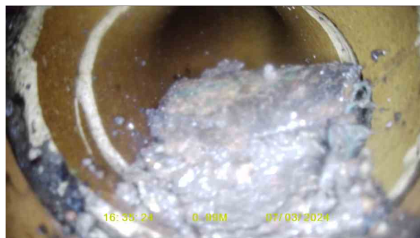
RWDP 7X_4de7d4eb-8b0c-4540-b134-49188c4c8bde_20240320_13 2813_237.jpg, 00:00:26, 0.99 m Fracture, multiple at joint from 12 o'clock to 12 o'clock
