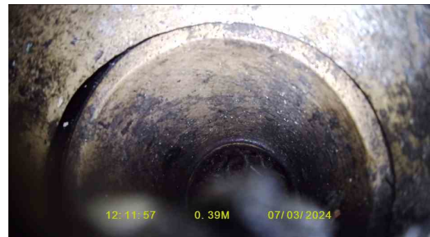
Red.Gully1X_284b2ead-1883-4418-9efe-a9f249573e7c_20240319_154140_751.jpg, 00:00:20, 0.39 m Open joint, medium
