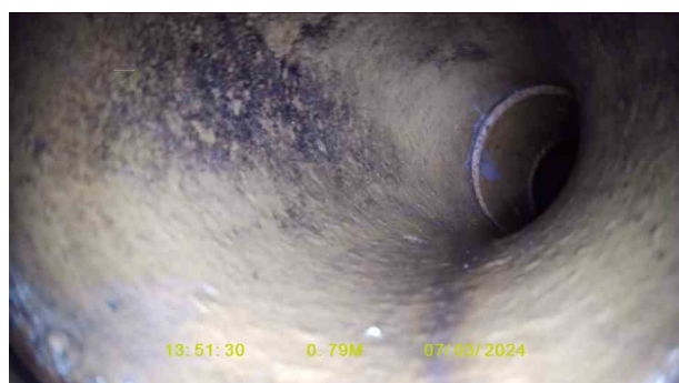
Gully 1X_913665fd-2640-4e67-b9ce-91c4f60e597c_20240320_102 341_246.jpg, 00:00:23, 0.79 m Line deviates right
