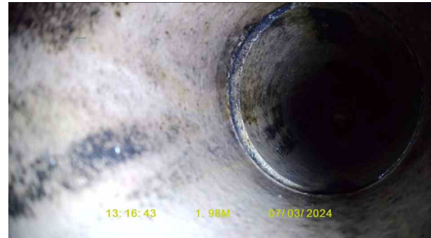
RWDP 5X_3513b94c-a5cf-44b8-ab46-8533a9c5dd41_20240320_084 608_577.jpg, 00:00:47, 1.98 m Open joint, medium
