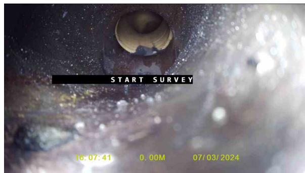
Manhole 10X_2ac0b7c4-a544-4421-adf7-bcacb684004c_20240320_13 5300_970.jpg, 00:00:02, 0.00 m Water level, 0% of the vertical dimension
