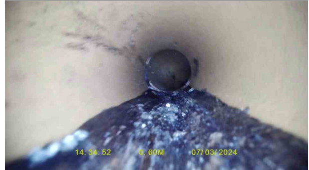
Manhole 5X_3f23308d-15b8-4f79-88ec-e9cb87715556_20240320_111 522_771.jpg, 00:00:16, 0.60 m Settled deposits, coarse, 10% cross-sectional area loss
