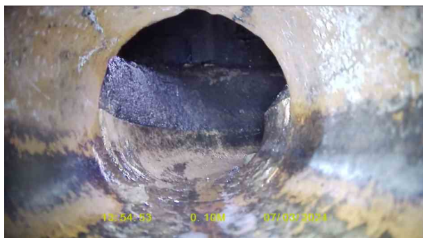
Manhole 3X_74ec6c76-09a0-4968-a7fd-79c163981c3e_20240320_103 722_672.jpg, 00:00:13, 0.10 m Line deviates right
