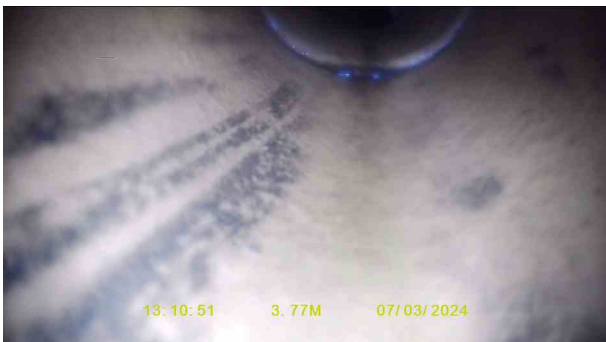
RWDP 3X_bd00792f-c217-433f-8a7e-ae7f67bbce1e_20240319_1641 34_207.jpg, 00:00:47, 3.77 m Line deviates up
