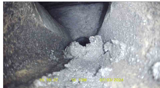
Manhole 7X_4631b8ee-d8a7-41d9-aef7-febc9e868cdd_20240320_125 256_481.jpg, 00:01:43, 10.10 m Settled deposits, fine, 15% cross-sectional area loss
