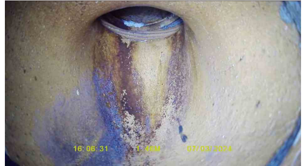
RedundantX_0855396a-043d-45f7-ac83-5b960e2d9bb7_2024 0320_135030_087.jpg, 00:00:33, 1.46 m Line deviates up, Rest Bend
