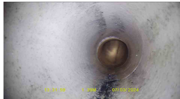
RWDP 6X_1651bdb6-0acb-4e87-a5f2-7ff06c594d64_20240320_0943 22_436.jpg, 00:00:59, 1.39 m Crack, circumferential from 2 o'clock to 6 o'clock
