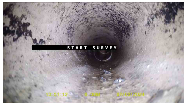
Gully 1X_41f2f058-b35d-4f7a-9dfd-b0af0b8541fe_20240320_10224 4_456.jpg, 00:00:05, 0.00 m Water level, 0% of the vertical dimension
