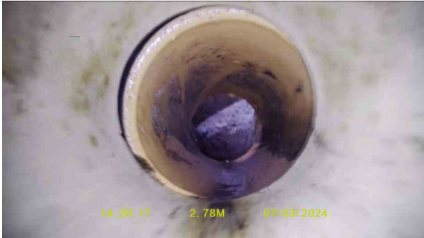
Manhole 4X_cf104af0-a512-4305-bd94-7e1f9818d2d6_20240320_1045 47_211.jpg, 00:00:49, 2.78 m Open joint, medium
