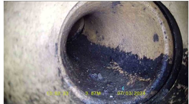
Gully 1X_b7f24a29-3480-45ed-9ae3-af38404f719a_20240320_102 758_513.jpg, 00:01:16, 3.87 m Open joint, large
