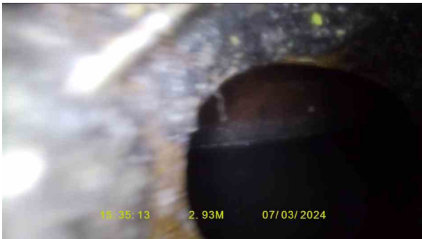
Manhole 9X_24c0d3f5-80ff-4a2a-b965-53c5cd5ef516_20240320_1319 13_907.jpg, 00:01:26, 2.93 m General remark, Drops into main line via junction
