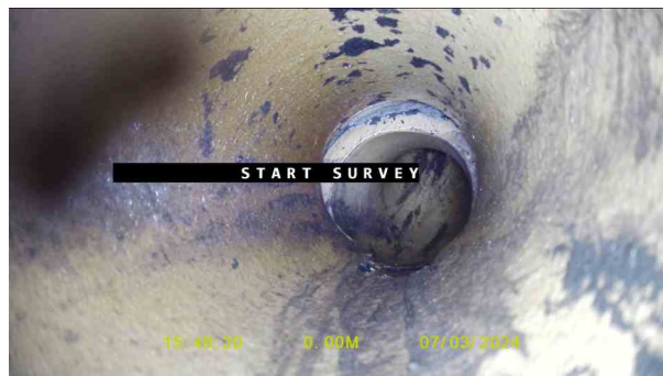
RedundantX_10747301-0ddb-4567-a807-511cebf3667b_2024 0320_134226_478.jpg, 00:00:03, 0.00 m Water level, 0% of the vertical dimension
