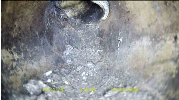
SVP 5X_79afa480-b583-46b9-a2de-ba887e197790_20240320_11 2311_885.jpg, 00:00:57, 3.47 m Line deviates up, Rest Bend
