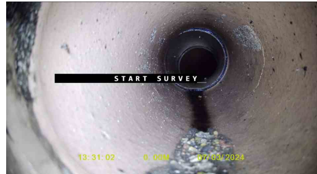
RWDP 6X_f1ad8b92-2450-4fe7-b439-f8d238a0a976_20240320_093 623_347.jpg, 00:00:02, 0.00 m Water level, 0% of the vertical dimension
