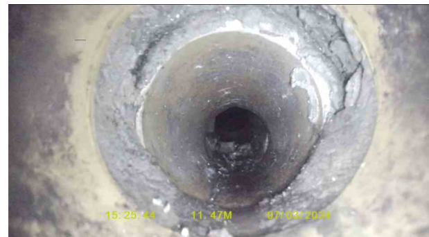
Manhole 8X_72bfa4cb-2bd6-42bc-870b-6ab8eb562af6_20240320_130 852_380.jpg, 00:02:20, 11.47 m Open joint, large
