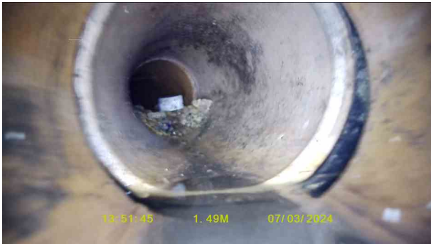
Gully 1X_ce571131-df52-4d57-822c-c7a8c5ad5515_20240320_102 503_528.jpg, 00:00:38, 1.49 m Open joint, large
