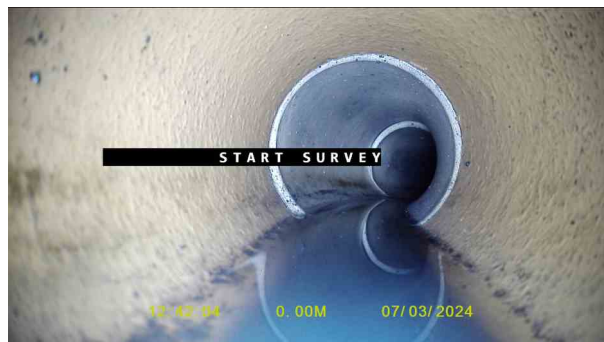
Manhole 1X_b684a182-9460-4678-a955-c75f56a6457b_20240319_162 416_487.jpg, 00:00:03, 0.00 m Water level, 5% of the vertical dimension
