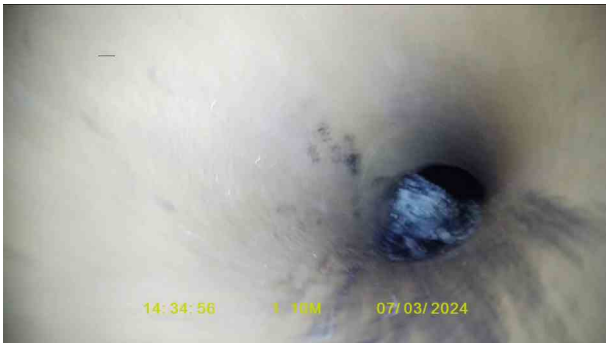
Manhole 5X_56eb968e-8c13-4651-a0f5-145292a4b94e_20240320_111 540_066.jpg, 00:00:20, 1.10 m Line deviates right
