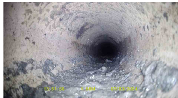
Gully 1X_f2b99e48-db12-4270-8dcd-34b28e4c4d14_20240320_102 654_591.jpg, 00:00:51, 1.93 m Settled deposits, fine, 10% cross-sectional area loss
