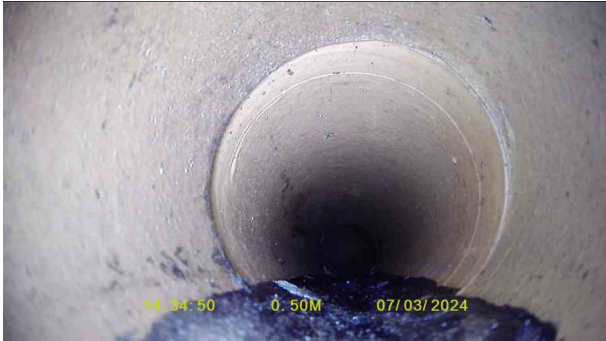
Manhole 5X_b64fad70-cb31-407c-a04b-6266f652e273_20240320_111 413_547.jpg, 00:00:14, 0.50 m Crack, circumferential from 8 o'clock to 4 o'clock
