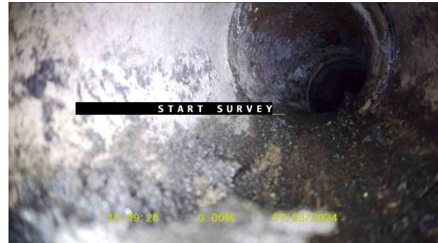
RedundantX_8508ad4d-1b92-4589-b3f0-3d895807bf94_2024 0320_124549_081.jpg, 00:00:03, 0.00 m Water level, 0% of the vertical dimension
