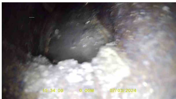
Manhole 9X_9d39f0eb-aa45-4037-846e-71f5da7da15f_20240320_131357_401.jpg, 00:00:13, 0.06 m General remark, Drops into main channel
