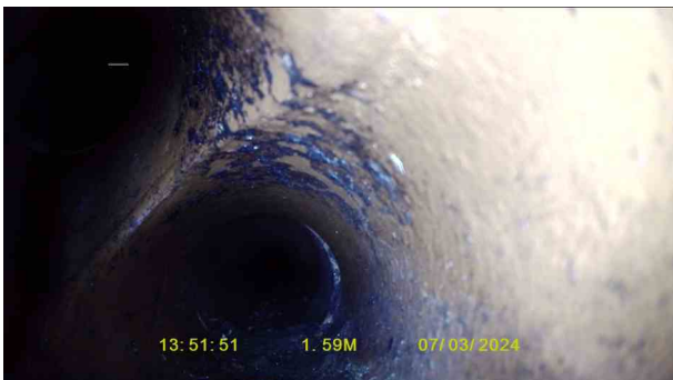
Gully 1X_699bef15-4056-4fa3-b40e-d84956fbfb8c_20240320_1026 27_547.jpg, 00:00:44, 1.59 m Defective junction, damaged at 10 o'clock, diameter: 100mm
