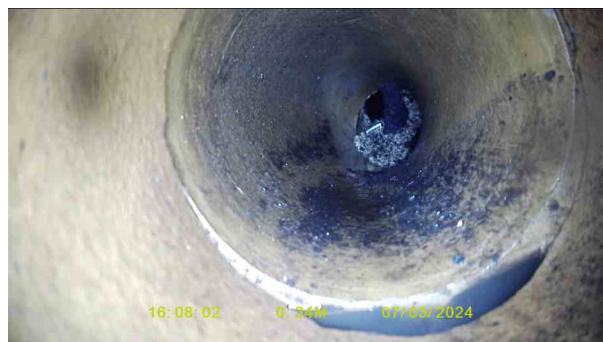
Manhole 10X_06eaf6d7-a0e7-4971-8a16-8103644500ac_20240320_13 5420_600.jpg, 00:00:23, 0.40 m Open joint, medium
