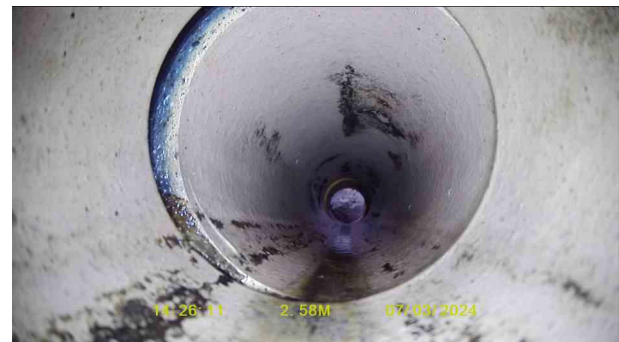
Manhole 4X_33011e05-1a2d-476f-8880-bcb86fc60f80_20240320_104427_334.jpg, 00:00:43, 2.58 m Open joint, medium
