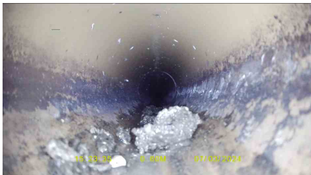
Manhole 8X_de174dfa-a69e-437a-aa01-28f535455762_20240320_125 546_643.jpg, 00:00:12, 0.47 m Settled deposits, coarse, 10% cross-sectional area loss
