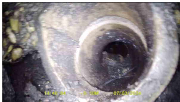
Manhole 6X_a757fd52-7cfa-4a75-8ecd-5504444e4bf1_20240320_1237 19_371.jpg, 00:00:14, 0.10 m Collapsed drain or sewer
