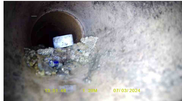
Gully 1X_56dbc946-710d-462b-b4e0-fb8535b12485_20240320_102 558_250.jpg, 00:00:41, 1.50 m Settled deposits, coarse, 15% cross-sectional area loss
