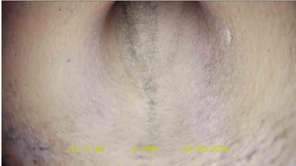
RWDP 5X_e9d00c25-dfd7-415e-8d43-ba3a9e961f53_20240320_085 124_508.jpg, 00:01:04, 2.78 m Line deviates up, Rest Bend
