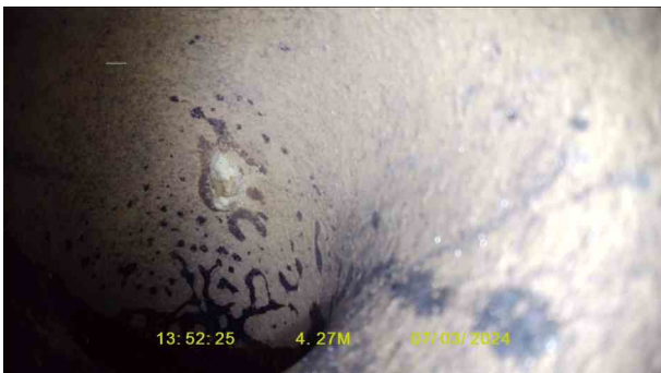
Gully 1X_fb08b2d2-a9f9-436d-bd3c-e0fa9a2c2510_20240320_1029 22_567.jpg, 00:01:18, 4.27 m Finish node, gully, reference: Gully 1
