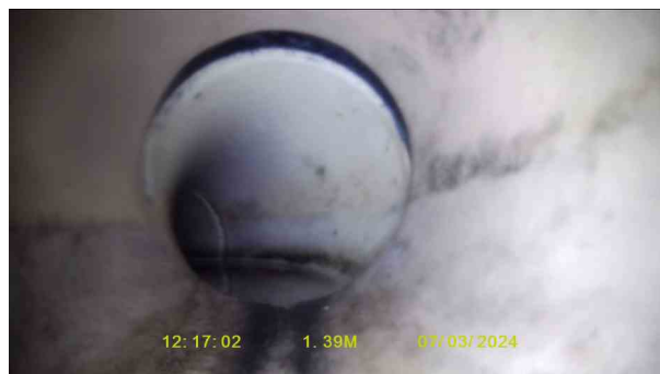
RWDP 2X_fa8ba669-2d8f-4e0b-81e0-f33b2e3c24cb_20240319_1549 11_092.jpg, 00:00:26, 1.38 m Open joint, medium
