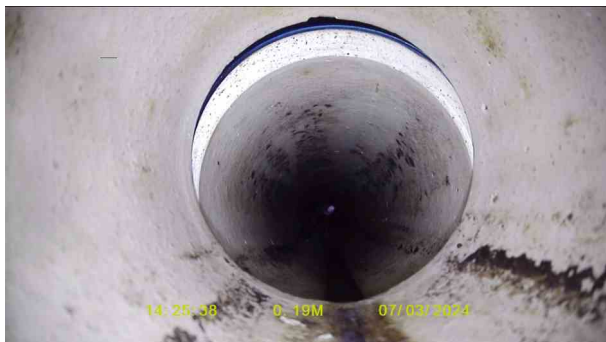
Manhole 4X_4bd82246-b6d0-42a2-a844-e36aa7aeacc7_20240320_104337_194.jpg, 00:00:10, 0.19 m Joint displaced, large
