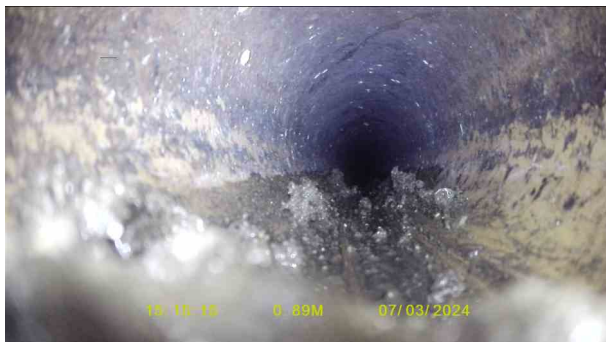
Manhole 7X_4cc60a64-7052-48d9-8096-f8aa2f18c6fa_20240320_1251 09_892.jpg, 00:00:22, 0.89 m Settled deposits, coarse, 10% cross-sectional area loss
