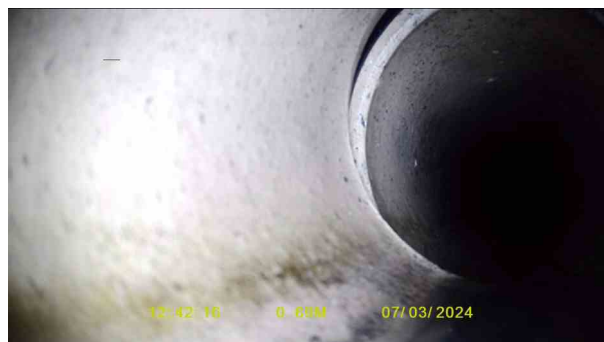
Manhole 1X_7bb2b75d-f8e4-46af-98ab-b3472451d36c_20240319_162 457_536.jpg, 00:00:16, 0.69 m Open joint, medium
