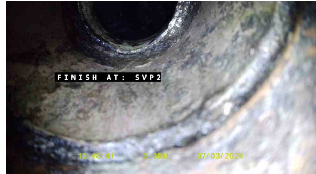
SVP 2X_ac865a6e-8d8f-4034-add3-ca4ed32e6d45_20240320_100 851_523.jpg, 00:00:34, 2.38 m Finish node, major connection without manhole, reference: SVP 2
