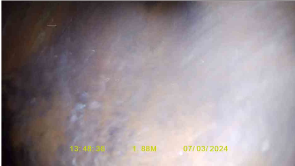
SVP 2X_1853355a-2981-4dec-9ee5-243edb5a1210_20240320_10 0833_328.jpg, 00:00:30, 1.88 m Line deviates up, Rest Bend
