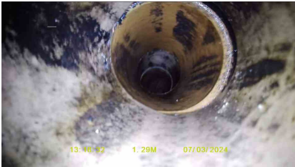
RWDP 5X_8e1fdab9-3f0d-4725-9729-8bc467dd17ad_20240320_084 524_241.jpg, 00:00:36, 1.29 m Open joint, medium
