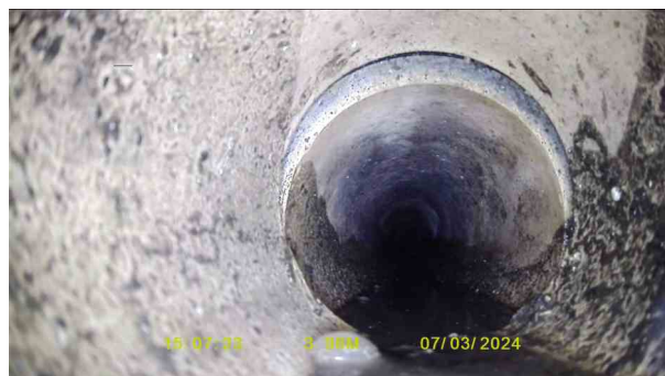
SVP 7X_0f50c5e0-7b5b-47e4-bf2e-5a8a5dffc9bf_20240320_12430 3_784.jpg, 00:01:12, 3.98 m Open joint, medium
