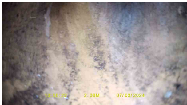
SVP 3X_8c09b435-3ca2-4c57-881b-727da00f3e23_20240320_102 039_070.jpg, 00:00:50, 2.38 m Line deviates up, Rest Bend
