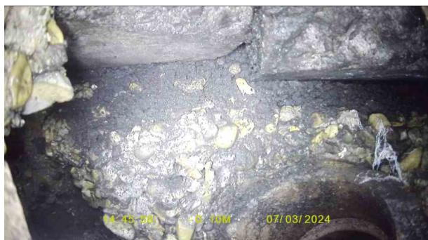
Manhole 6X_fb349593-b3ee-4de9-bb3f-f9efa26295b7_20240320_1236 05_857.jpg, 00:00:08, 0.10 m Void visible beyond defect
