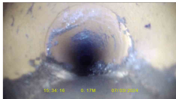
Manhole 9X_db496bb9-53d4-446d-9bc7-6258fdb40230_20240320_131438_318.jpg, 00:00:29, 0.17 m Attached deposits, encrustation from 5 o'clock to 9 o'clock, 15% cross-sectional area loss
