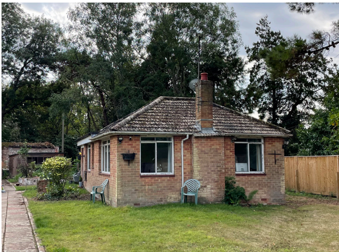
Existing bungalow in disrepair
