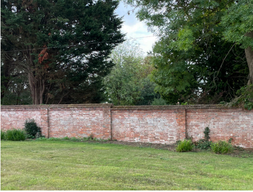
4 - The eastern half of the southern boundary wall was demolished and then rebuilt to match the existing due to structural collapse. This wall falls within the site boundary.
