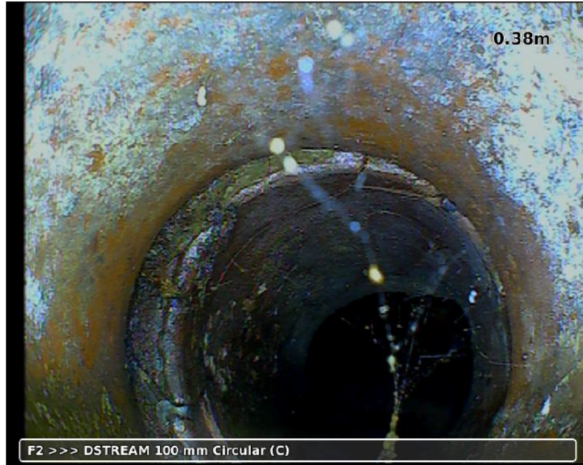
Photo: 20230130-083451-snap0002.jpg, 00:00:47 0.38m, Cracks multiple at joint from/at 07 o'clock to 02 o'clock
