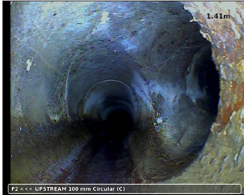
Photo: 20230130-083212-snap0002.jpg, 00:00:26 1.41m, Junction from/at 02 o'clock diameter: 100 mm
