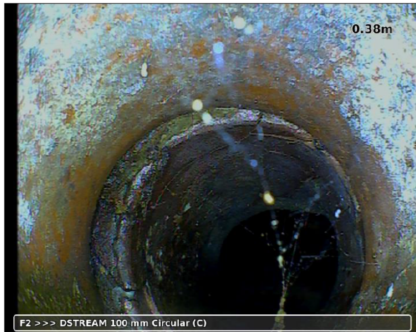
Photo: 20230130-083451-snap0001.jpg, 00:00:35 0.38m, Joint displaced medium
