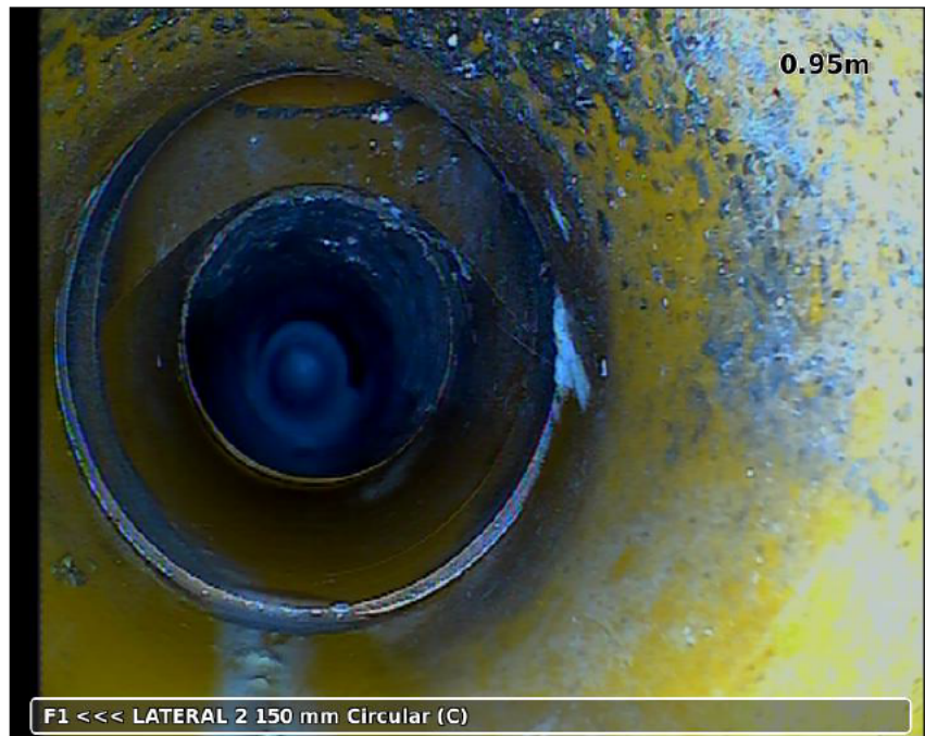
Photo: 20230130-082500-snap0001.jpg, 00:00:29 0.95m, Junction from/at 12 o'clock diameter: 100 mm
