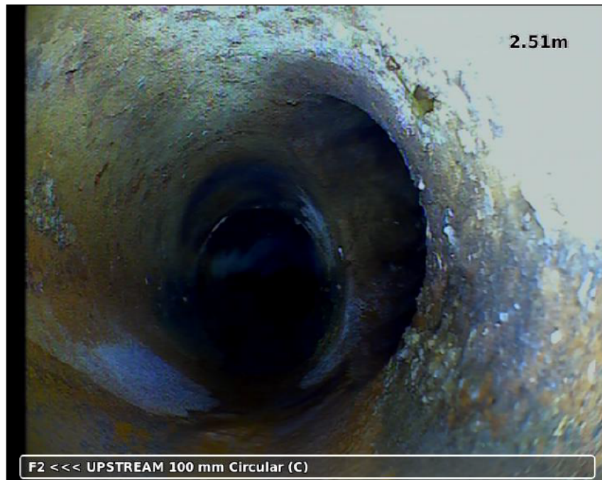
Photo: 20230130-083212-snap0003.jpg, 00:01:01 2.51m, Junction from/at 02 o'clock diameter: 100 mm
