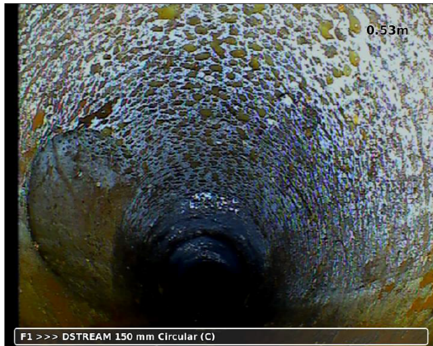
Photo: 20230130-082748-snap0001.jpg, 00:00:25 0.53m, Junction from/at 10 o'clock diameter: 100 mm
