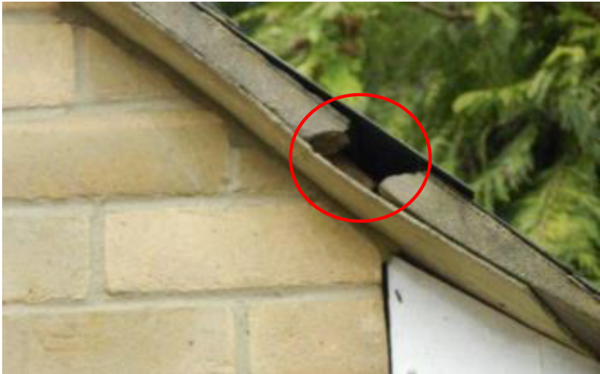
Image 11 – Deterioration to the North elevation of the garage/annex structure offering likely shelter/access opportunities for bats within
