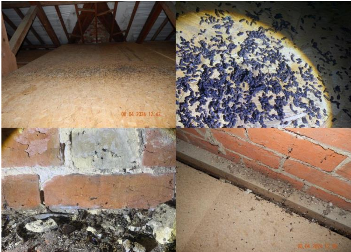
Image 7 – Evidence of 2000+ bat droppings observed within the main roof void spaces to the dwelling
