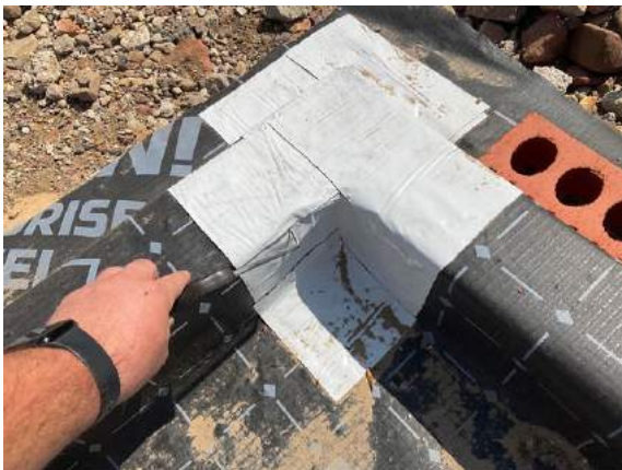
Plot 16. Pick test to sealed corner details.
