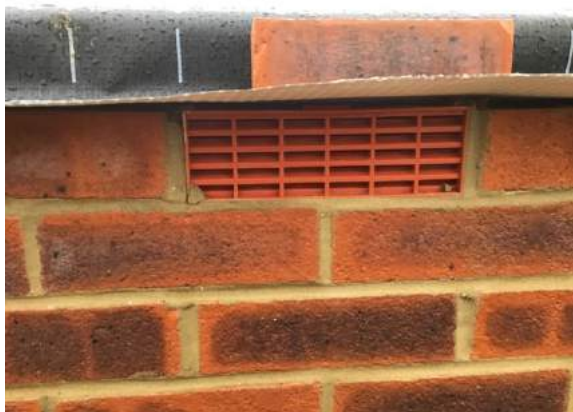
Air bricks were in place under the membrane to plots 31,36,77 & 78 at the time of our inspection.
