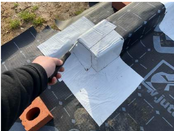
Plot 34. Pick testing upon sealed door threshold details.
