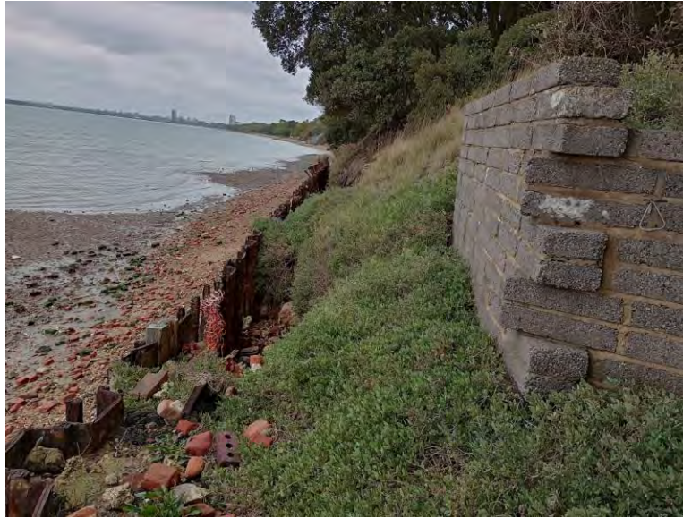
Figure 1: View looking north along the cliff face with eroded sheet piling below.
