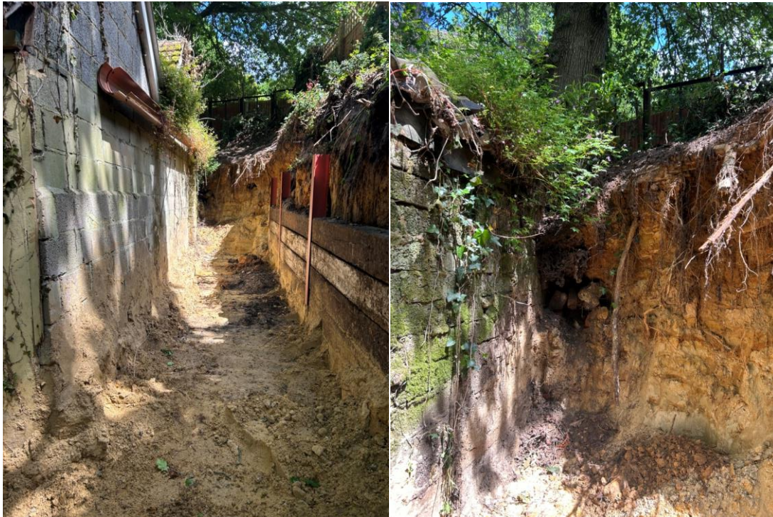
Figure 2: Photographs showing retaining wall to rear of garage and bank/roots collapsed against rear left corner.
