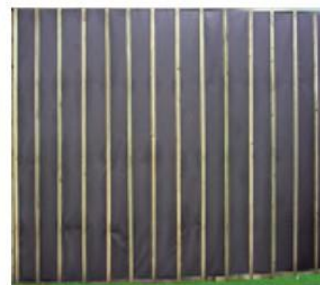
Rear view showing protective plastic membrane
