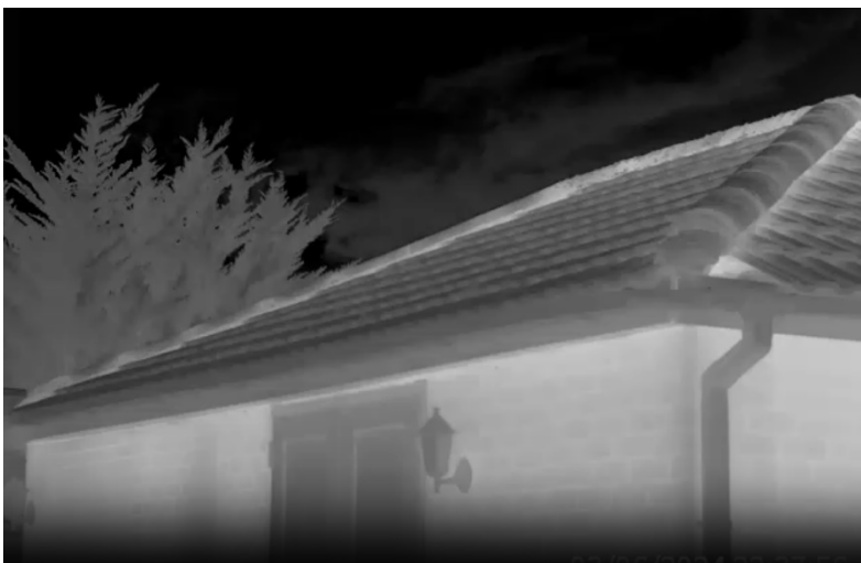
Figure 6. Field of view of 2 nd survey NVA (thermal camera) on southern corner of building. Image taken at darkest point of survey.
