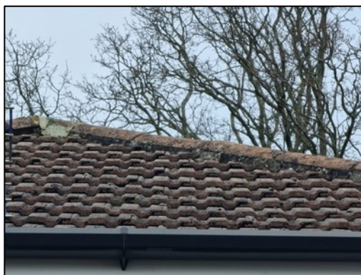
Figure 5 – lifted roof tiles on western roof face
