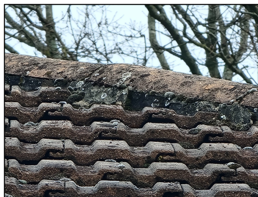
Figure 6 – lifted roof tiles
