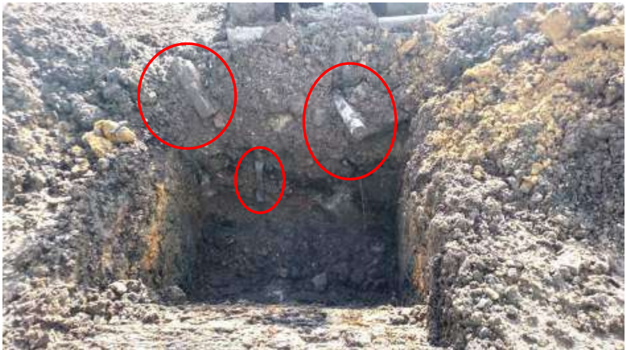
Photograph 6: Excavation in mixed soils stockpile – unsuitable materials circled
