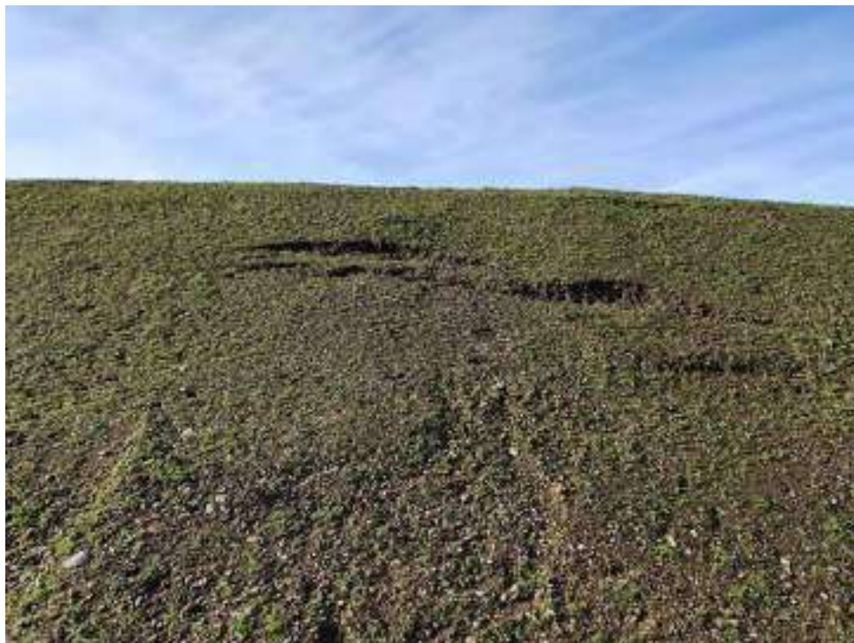
Photograph 4: Surface cracks in bund. Facing southwest.
