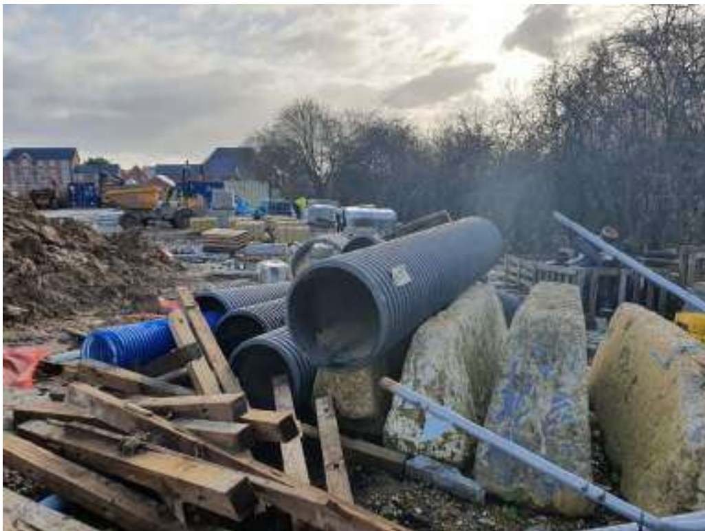
Photograph 2: Storage of general construction waste at southern most end of Burr ridge Green TS stockpile.
