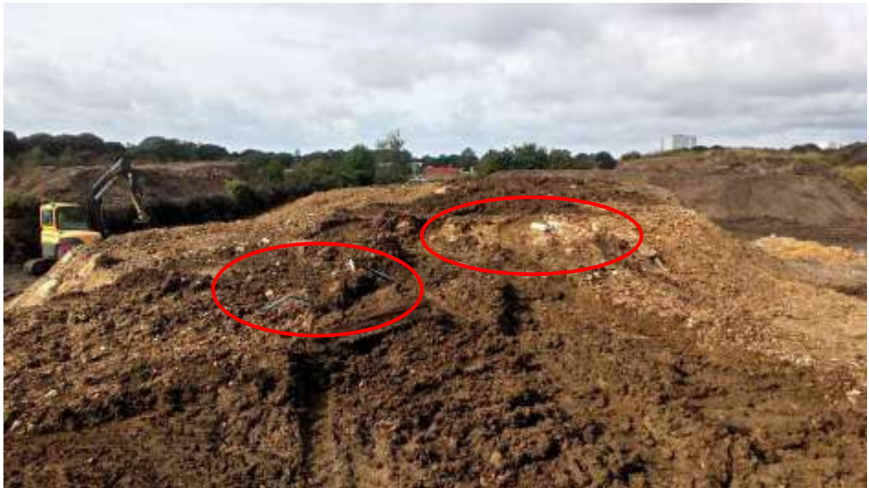
Photograph 5: Mixed soils stockpile – unsuitable materials circled
