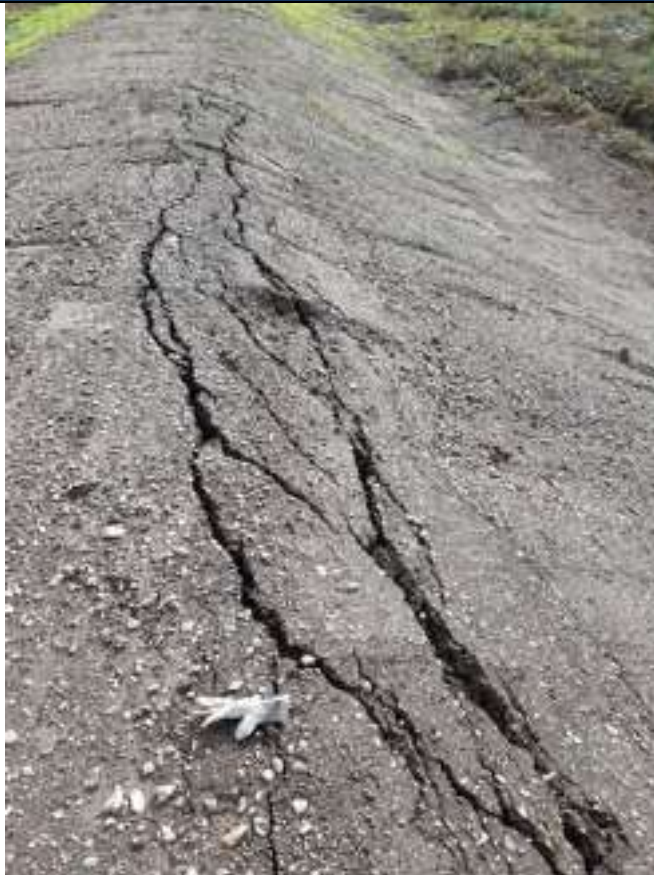
Photograph 3: Surface cracks within topsoil of the bund.
