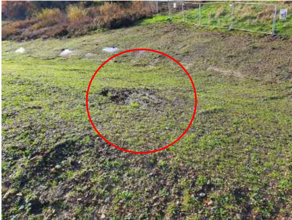
Photograph 5: Small bund failure on west facing slope of bund (approx. 2m length)
