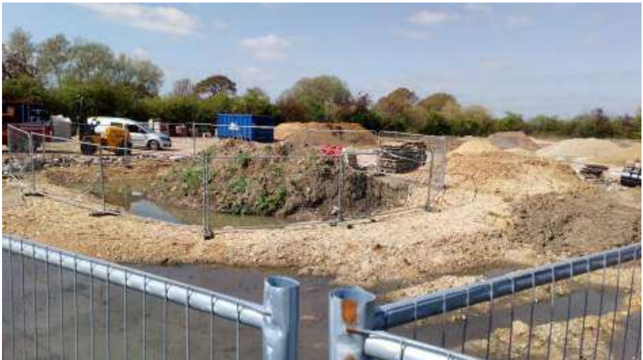
Photograph 4: Asbestos impacted materials fenced off and various aggregate stockpiles
