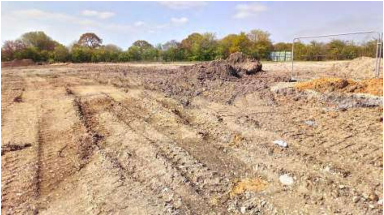
Photograph 6: View looking south west across Japanese Knotweed burial cell
