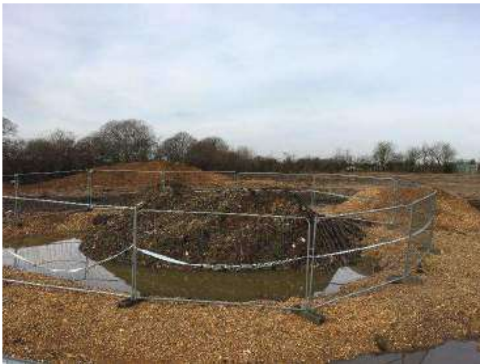
Photograph 6: asbestos impacted soils remain on site following completion of knotweed remediation
