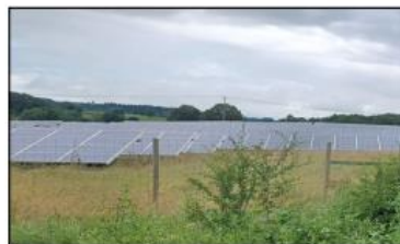
Example Panels and Security fencing
