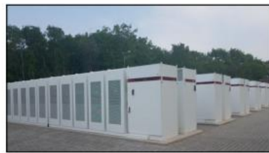
Example Battery Units
