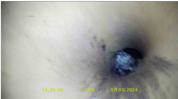
Manhole 5X_56eb968e-8c13-4651-a0f5-145292a4b94e_20240320_111 540_066.jpg, 00:00:20, 1.10 m Line deviates right
