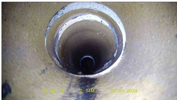
RedundantX_560928bb-2841-4d01-9e39-9ce7daa3e46d_202 40320_134924_385.jpg, 00:00:15, 0.34 m Open joint, large
