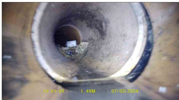
Gully 1X_ce571131-df52-4d57-822c-c7a8c5ad5515_20240320_102 503_528.jpg, 00:00:38, 1.49 m Open joint, large
