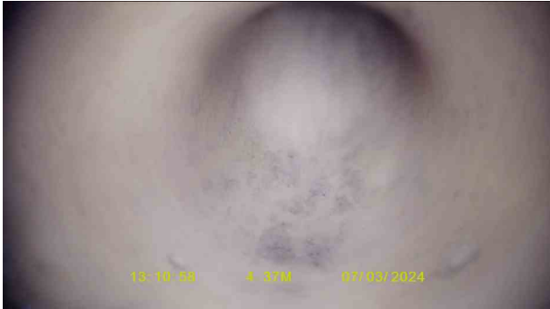
RWDP 3X_ccf954a8-0561-48b4-8ef0-9151b7da0c65_20240319_164 223_998.jpg, 00:00:54, 4.37 m Line deviates up, Rest Bend
