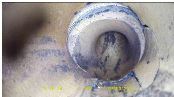
RedundantX_df7325ca-5cf0-495b-8a73-e4da87f2bfc5_20240 320_134254_147.jpg, 00:00:08, 0.02 m Broken pipe from 2 o'clock to 7 o'clock
