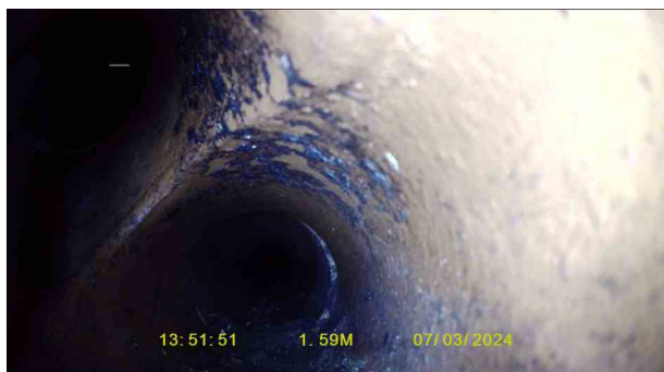
Gully 1X_699bef15-4056-4fa3-b40e-d84956fbfb8c_20240320_1026 27_547.jpg, 00:00:44, 1.59 m Defective junction, damaged at 10 o'clock, diameter: 100mm
