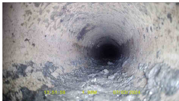
Gully 1X_f2b99e48-db12-4270-8dcd-34b28e4c4d14_20240320_102 654_591.jpg, 00:00:51, 1.93 m Settled deposits, fine, 10% cross-sectional area loss
