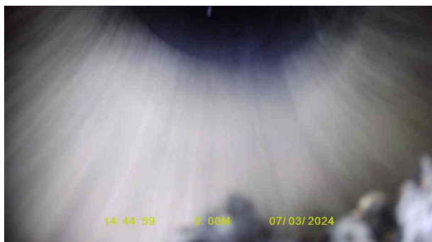
SVP 6X_94780432-1803-47ab-a24f-15b1bd62ac64_20240320_112 713_436.jpg, 00:00:07, 0.02 m Line deviates up, Rest Bend
