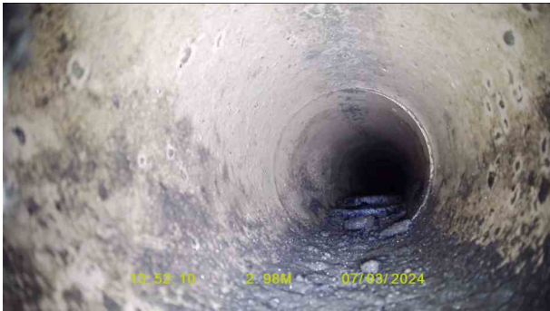
Gully 1X_4a890346-184e-48ea-aada-441c30087dbd_20240320_10 2722_748.jpg, 00:01:03, 2.98 m Line deviates right
