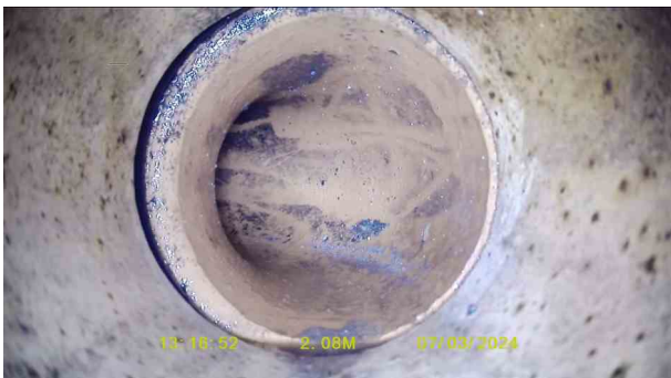
RWDP 5X_70f1eed3-d8d3-4af1-ab1c-c26661957663_20240320_084 631_783.jpg, 00:00:57, 2.08 m Open joint, medium
