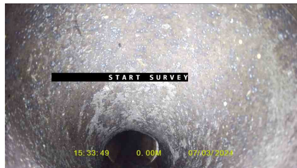
Manhole 9X_e7f38a73-21a8-4bad-9fe2-7e61806e3789_20240320_131 321_040.jpg, 00:00:03, 0.00 m Water level, 0% of the vertical dimension
