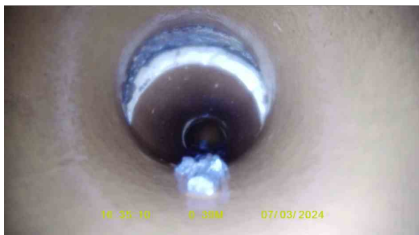
RWDP 7X_d0d7c3e2-48f9-4c71-9200-9e59110ae0e5_20240320_132 659_050.jpg, 00:00:12, 0.39 m Joint displaced, large
