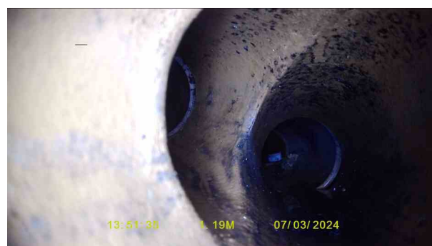
Gully 1X_6b781769-2e2b-4a2a-b658-b91de4cd7f0c_20240320_102 435_277.jpg, 00:00:28, 1.19 m Junction at 9 o'clock, diameter: 100mm
