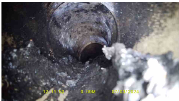
Red.Gully1X_1c9f7630-78b9-4089-a67f-0beb4fd04bda_20240319_153801_569.jpg, 00:00:14, 0.09 m Settled deposits, coarse, 20% cross-sectional area loss
