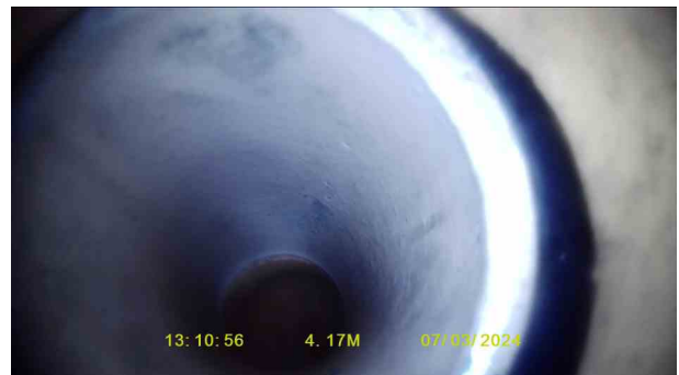
RWDP 3X_078e67e5-12dc-4ee0-9bfd-81994ebd52dc_20240319_164 158_713.jpg, 00:00:52, 4.17 m Open joint, large
