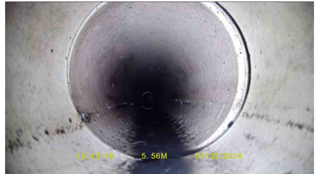
Manhole 1X_ac00c660-a1ef-4401-a0fe-c4bf8f745155_20240319_1628 48_159.jpg, 00:01:16, 5.56 m Open joint, medium
