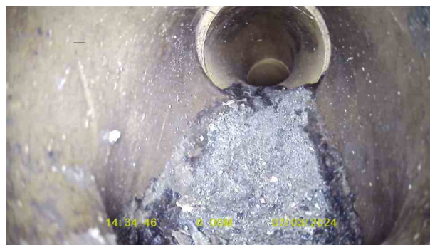
Manhole 5X_119f0b8f-6544-4a8a-a0b1-066a48cf28c2_20240320_1114 55_101.jpg, 00:00:10, 0.25 m General remark, Back of interceptor is cracked
