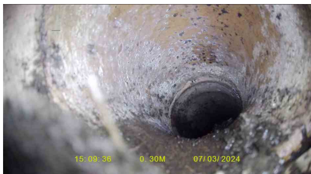
RedundantX_bfcb4812-3e59-4124-8a38-283a3c0081ef_2024 0320_124609_171.jpg, 00:00:11, 0.30 m Line deviates right
