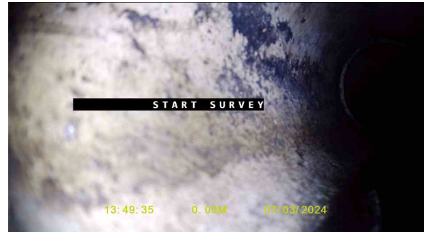
SVP 3X_4c4a2141-899f-474a-8b49-c8e07a04d1b4_20240320_101 030_571.jpg, 00:00:03, 0.00 m Water level, 0% of the vertical dimension
