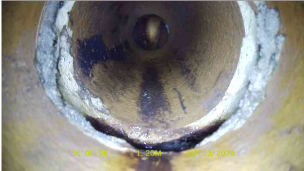
RedundantX_b57be1dc-841a-45df-9221-9fad4aa04acc_2024 0320_135006_143.jpg, 00:00:27, 1.20 m Void visible beyond defect
