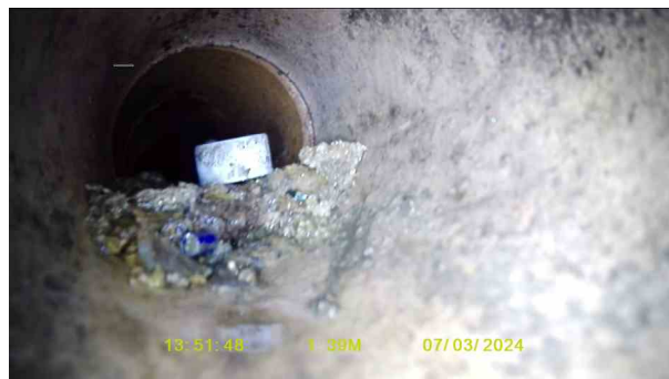
Gully 1X_56dbc946-710d-462b-b4e0-fb8535b12485_20240320_102 558_250.jpg, 00:00:41, 1.50 m Settled deposits, coarse, 15% cross-sectional area loss
