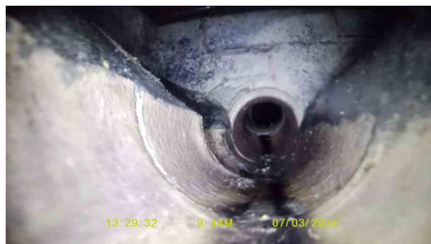
Buried MHX_52ddf933-9a3c-472f-bfcc-188da3222a8e_20240319_172707_457.jpg, 00:01:46, 9.54 m Finish node, manhole, reference: Buried MH
