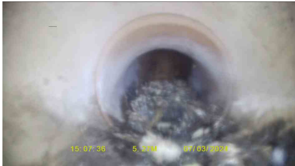
SVP 7X_d92e0fec-d581-491d-bf6a-4a85e52dd0c3_20240320_124 337_035.jpg, 00:01:26, 5.27 m Settled deposits, coarse, 15% cross-sectional area loss
