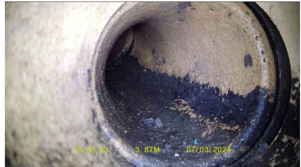
Gully 1X_b7f24a29-3480-45ed-9ae3-af38404f719a_20240320_102 758_513.jpg, 00:01:16, 3.87 m Open joint, large
