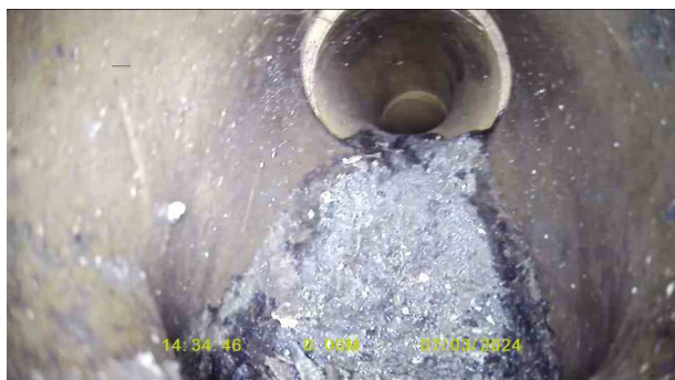
Manhole 5X_58e5fa59-be5e-434e-8fd9-ab32cc1e031b_20240320_111 348_530.jpg, 00:00:10, 0.10 m General remark, Drops into main channel
