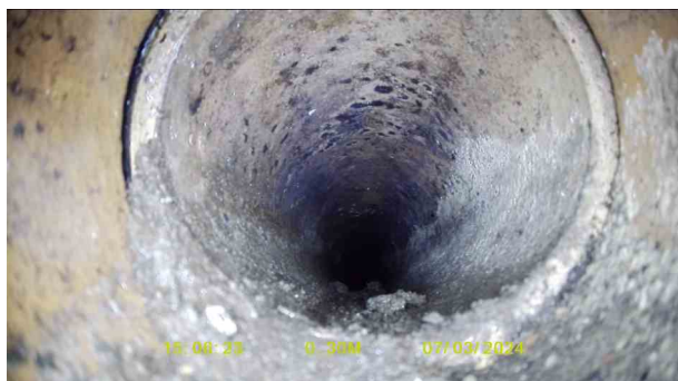
SVP 7X_efdaccdd-08b8-4519-a31f-c7a016f1bbbc9_20240320_1241 50_253.jpg, 00:00:13, 0.30 m Open joint, medium
