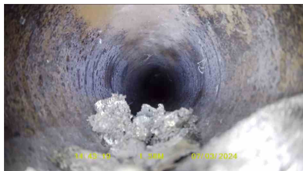
SVP 5X_c7001d65-6fa7-4f87-af60-9f809919c3db_20240320_1121 26_446.jpg, 00:00:33, 1.58 m Settled deposits, coarse, 10% cross-sectional area loss
