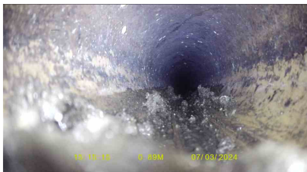
Manhole 7X_4cc60a64-7052-48d9-8096-f8aa2f18c6fa_20240320_1251 09_892.jpg, 00:00:22, 0.89 m Settled deposits, coarse, 10% cross-sectional area loss
