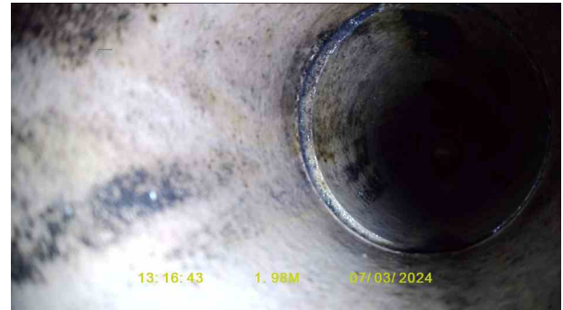
RWDP 5X_3513b94c-a5cf-44b8-ab46-8533a9c5dd41_20240320_084 608_577.jpg, 00:00:47, 1.98 m Open joint, medium
