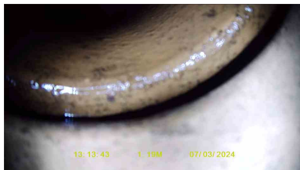
RWDP 4X_f5d31879-6314-4b1d-bd5e-a7c18aba2ff8_20240319_1710 26_337.jpg, 00:00:20, 1.19 m Open joint, medium
