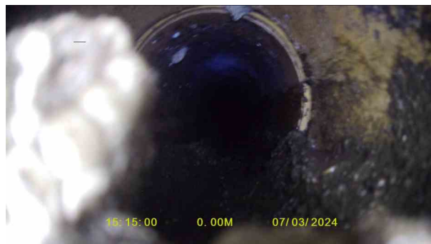
Manhole 7X_30993bdc-1365-4001-bb12-cc31c7f3c08d_20240320_125 040_456.jpg, 00:00:07, 0.00 m Water level, 0% of the vertical dimension
