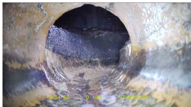
Manhole 3X_74ec6c76-09a0-4968-a7fd-79c163981c3e_20240320_103 722_672.jpg, 00:00:13, 0.10 m Line deviates right
