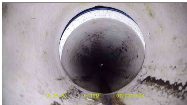
Manhole 4X_4bd82246-b6d0-42a2-a844-e36aa7aeacc7_20240320_104337_194.jpg, 00:00:10, 0.19 m Joint displaced, large
