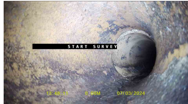
SVP 2X_26b65d00-1208-4d1e-a278-39bfca35a6a8_20240320_100 701_031.jpg, 00:00:04, 0.00 m Water level, 0% of the vertical dimension
