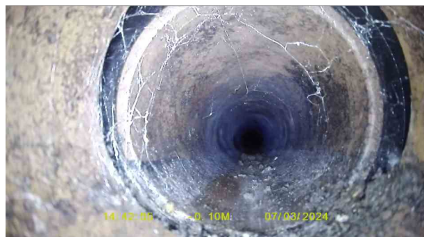
SVP 5X_39484c3e-6a53-41c7-8c2a-171520fb3b7e_20240320_112 028_103.jpg, 00:00:08, 0.10 m Open joint, large
