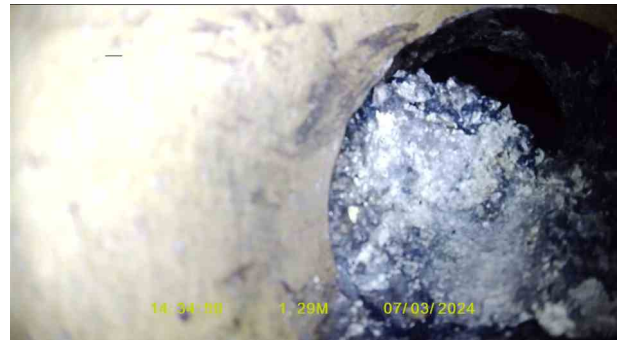
Manhole 5X_04b28b9d-c3d2-443d-8588-5e3fe19a8ddf_20240320_111 612_778.jpg, 00:00:23, 1.29 m Attached deposits, encrustation at joint from 4 o'clock to 10 o'clock, 35% cross-sectional area loss
