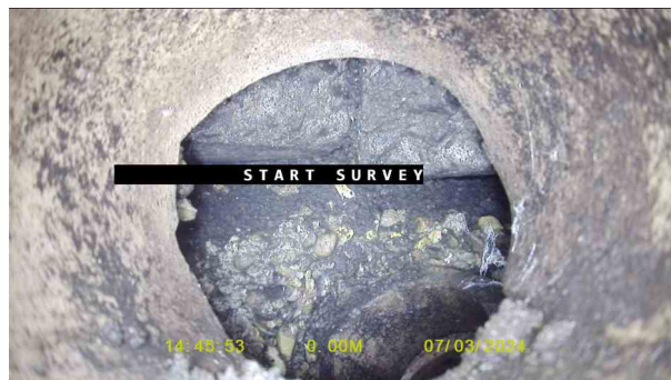
Manhole 6X_556df7d6-46b8-48eb-a9f1-8fc4b6b9461a_20240320_1130 04_585.jpg, 00:00:02, 0.00 m Water level, 0% of the vertical dimension
