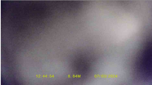
Manhole 1X_b7abf4c9-81f5-4a1f-beb7-38caa70de10f_20240319_163052_057.jpg, 00:02:18, 8.84 m Loss of vision, camera under water
