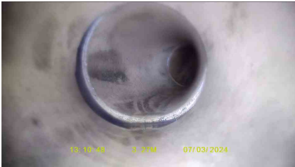
RWDP 3X_f5d68d39-689f-419d-aa9b-e6d821e21ac8_20240319_164 057_528.jpg, 00:00:44, 3.27 m Open joint, large
