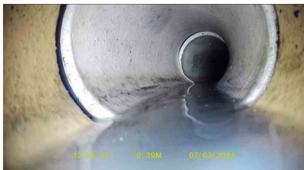
Manhole 1X_be6a1078-00da-4a70-9e33-1aae59830423_20240319_16 2437_590.jpg, 00:00:11, 0.39 m Open joint, medium
