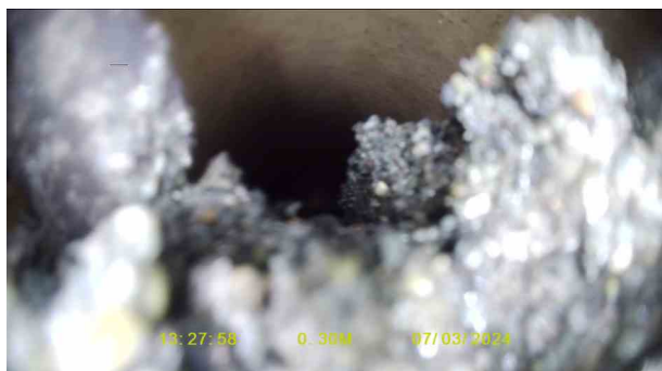
Buried MHX_39589844-ef90-42dc-84a6-54c9bb852f6f_20240319_172450_152.jpg, 00:00:12, 0.30 m Settled deposits, fine, 30% cross-sectional area loss
