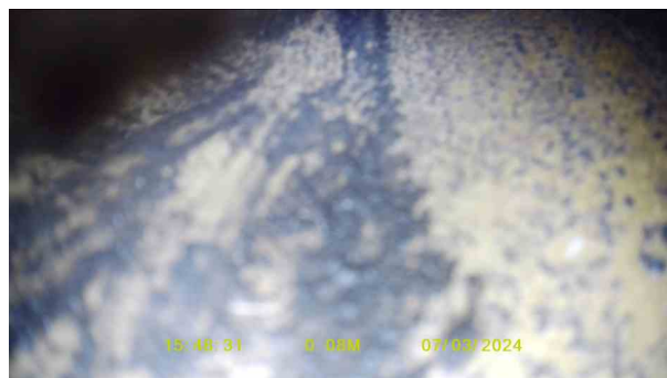
RedundantX_8665a7a0-298a-4a06-9f21-3be9d9540a98_2024 0320_134329_996.jpg, 00:00:14, 0.08 m Line deviates up, Rest Bend
