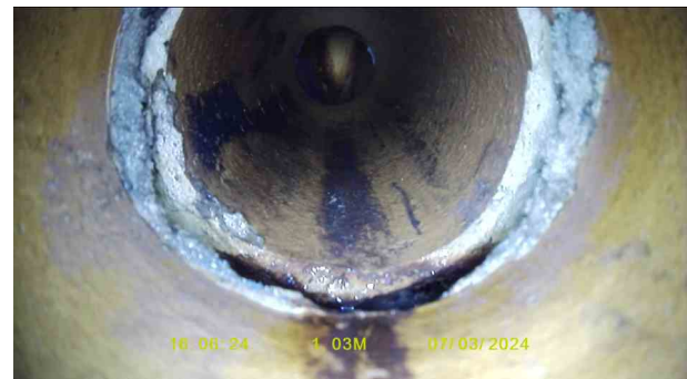
RedundantX_92cd8f92-8206-4401-ba8a-5e0bad02faff_20240 320_134948_097.jpg, 00:00:25, 1.03 m Open joint, medium
