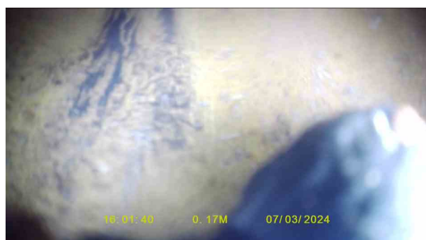
RedundantX_d158e46e-ebc0-42f9-8892-dd4de3553af9_2024 0320_134625_863.jpg, 00:00:07, 0.17 m Line deviates up, Rest Bend
