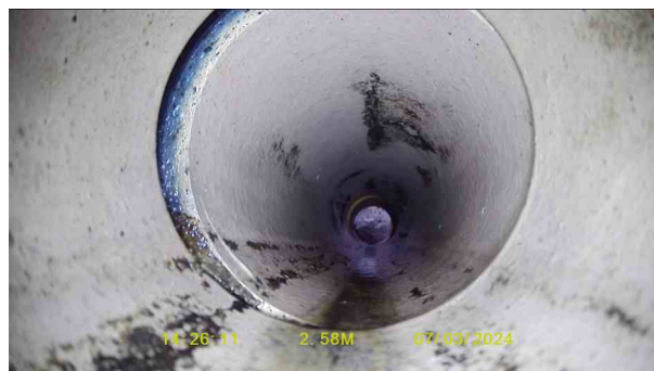
Manhole 4X_33011e05-1a2d-476f-8880-bcb86fc60f80_20240320_104427_334.jpg, 00:00:43, 2.58 m Open joint, medium
