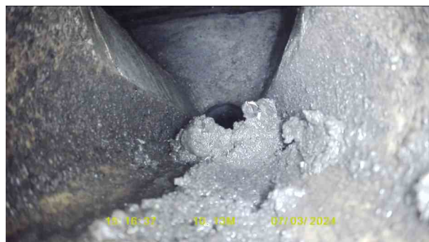
Manhole 7X_4631b8ee-d8a7-41d9-aef7-febc9e868cdd_20240320_125 256_481.jpg, 00:01:43, 10.10 m Settled deposits, fine, 15% cross-sectional area loss
