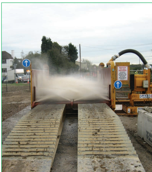
Figure 3.7 Wheel wash facility (courtesy Skanska)
