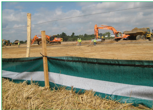
Figure 4.13 Wildlife Barriers (courtesy Skanska)
