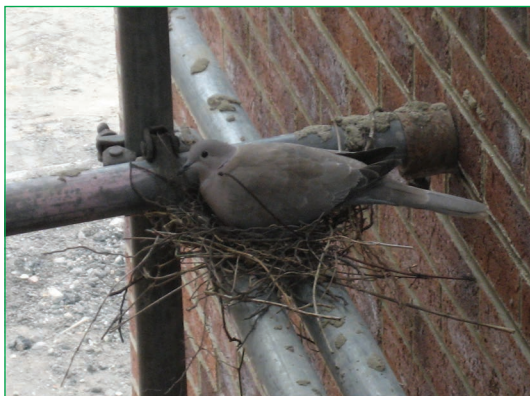
Figure 4.11 Bird nesting in scaffolding (courtesy Galliford Try plc)
