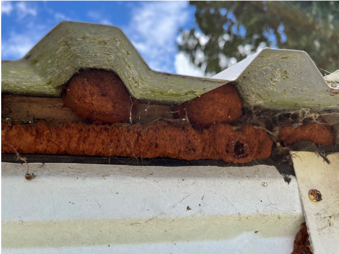
Figure 9 - image showing expanding foam in outbuilding roof
