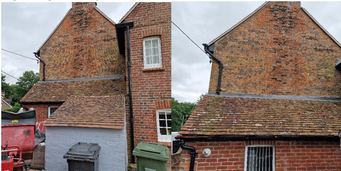
Photo 3: Two views of the small single-story roof, showing lifted tiles and small gaps
