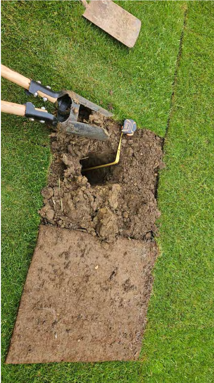
Photo of hole with tape in place
