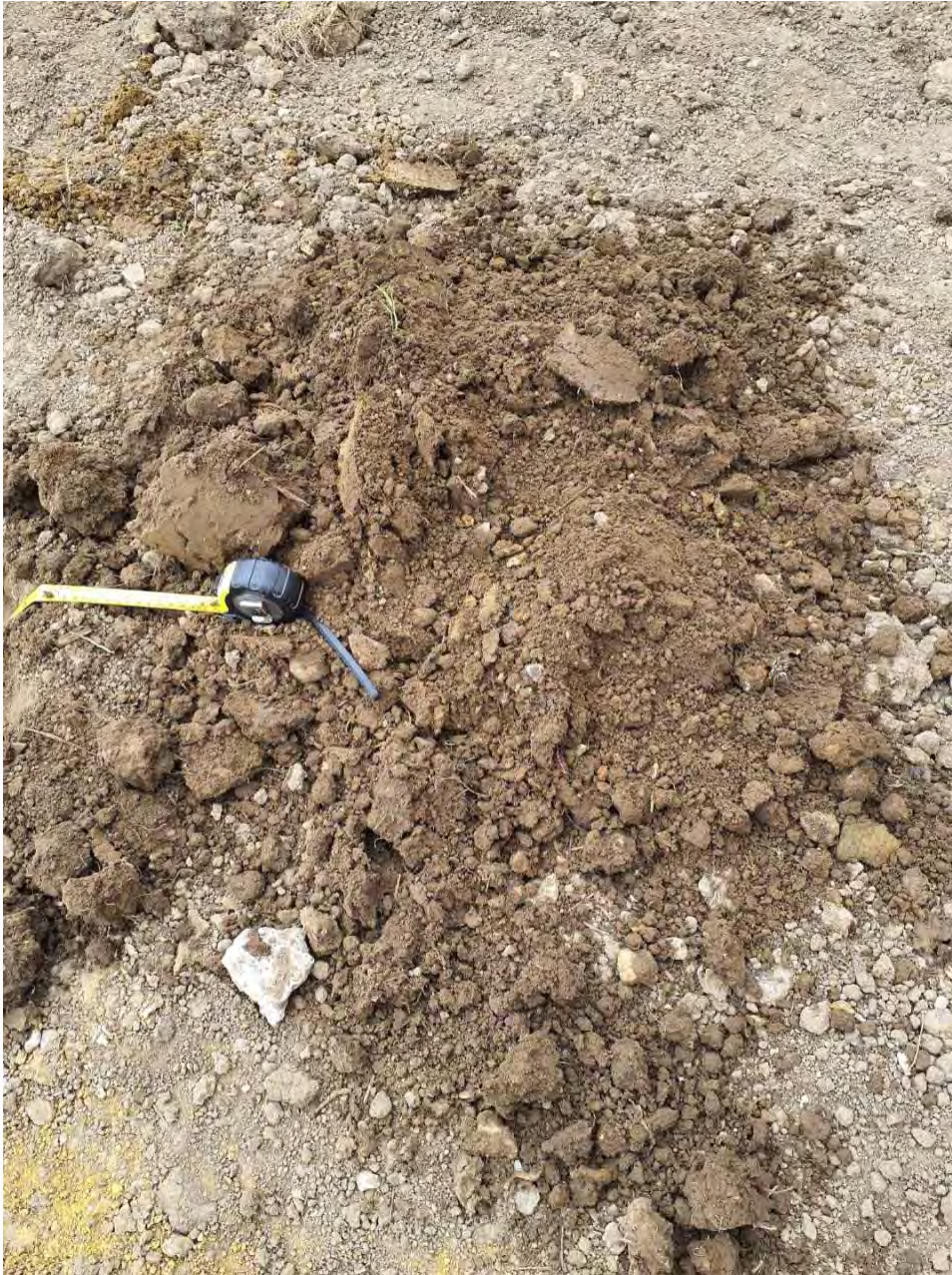
Photo of hole with tape in place
