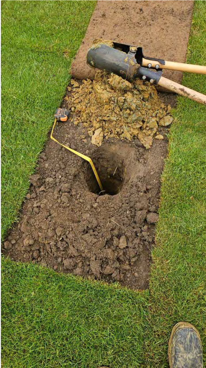
Photo of hole with tape in place
