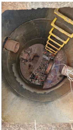
S24 UNABLE TO SURVEY THROUGH HYDRO BRAKE CONFINED SPACE REQUIRED_1
