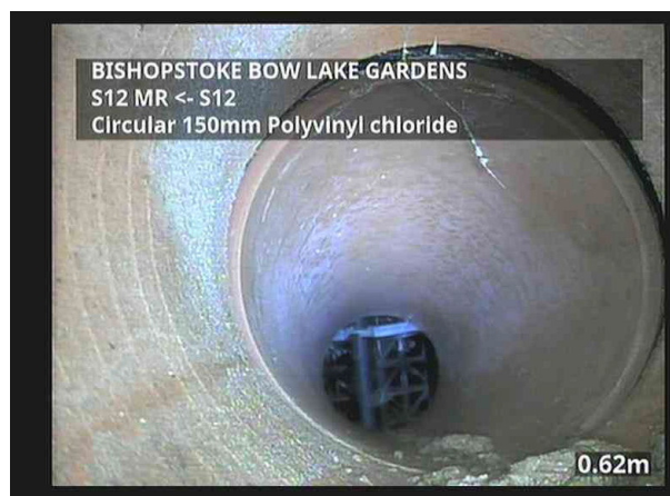
S12__TANK 2_2.jpg, 00:00:20, 0.62 m Open joint, medium
