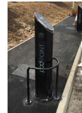
Electric Vehicle Charge Point
