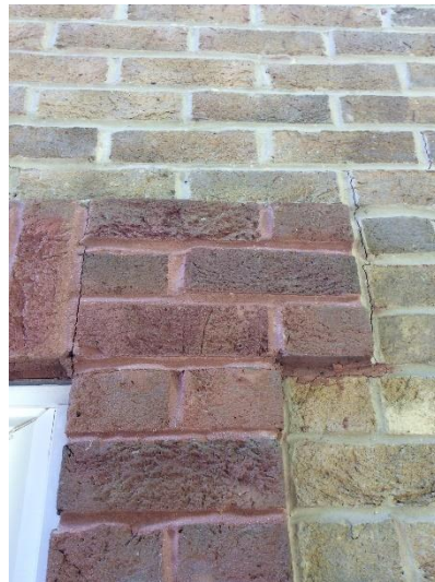
Picture 8: Cracking on left hand side of rear patio doors
