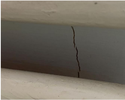
Picture 5: Vertical cracks noted around radiator beneath window in first floor bedroom on front right-hand side
