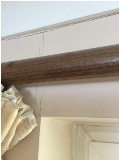
Picture 1: Very slight vertical cracking internally on left hand side above patio doors
