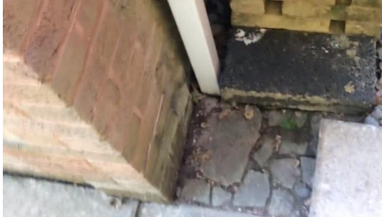
Picture 4: Rainwater down pipe located on rear left-hand corner, which appears to have dropped
