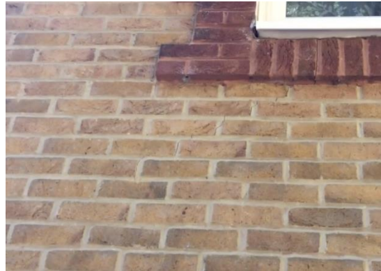
Picture 10: Diagonal crack above patio doors on rear left hand side going up to first floor bedroom window (with respective vertical internal cracking seen in picture 3)
