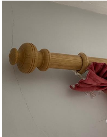
Picture 6: Cracks up to ceiling level near window in first floor bedroom on front right-hand side
