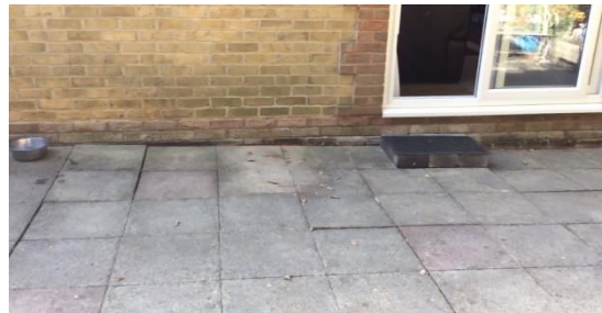
Picture 12: Patio paving slabs appear to have dropped towards rear left-hand corner (view 2)
