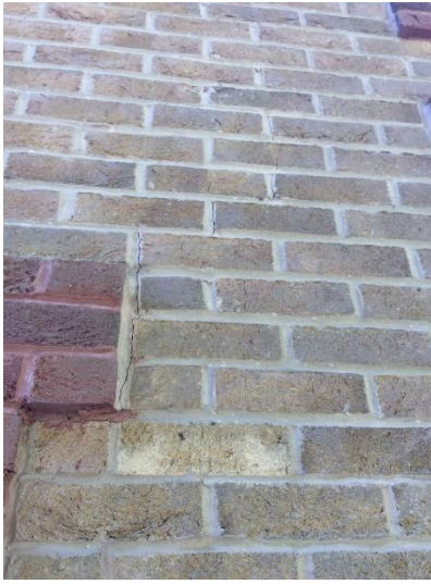
Picture 9: Diagonal crack extends up from left hand corner of rear left patio doors towards rear left corner
