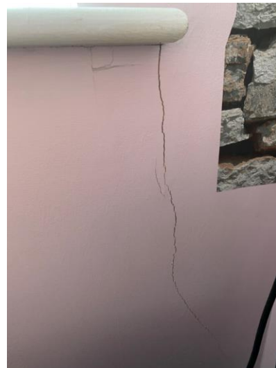
Picture 4: Vertical tapered cracking in first floor middle bedroom above the front door on left side of window
