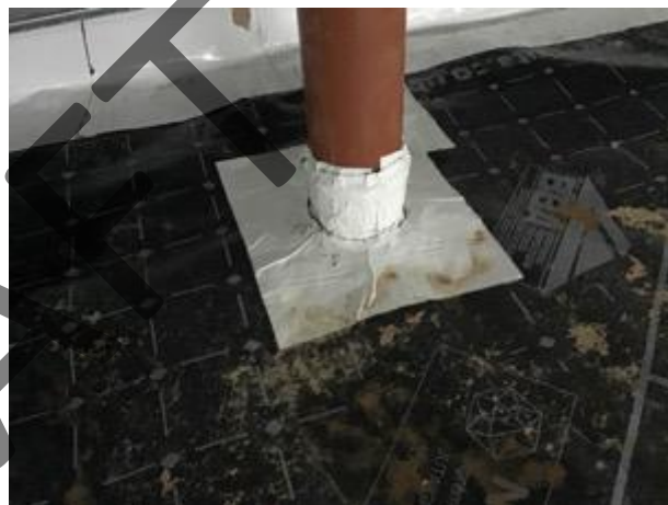
Typical pipe penetration seal using SAGM.
