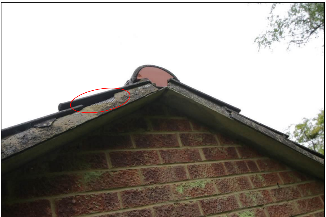
Photo 5: Gap in northern apex of garage may access a small roof cavity
