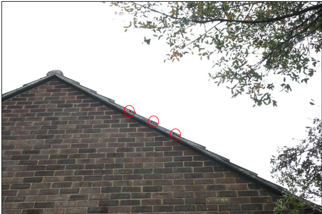
Photo 1: Small gaps present in apex of building
