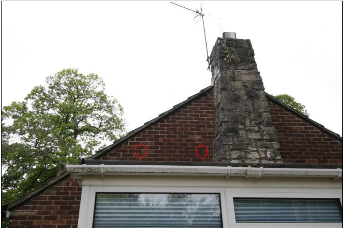
Photo 2: Small air gaps in apex wall
