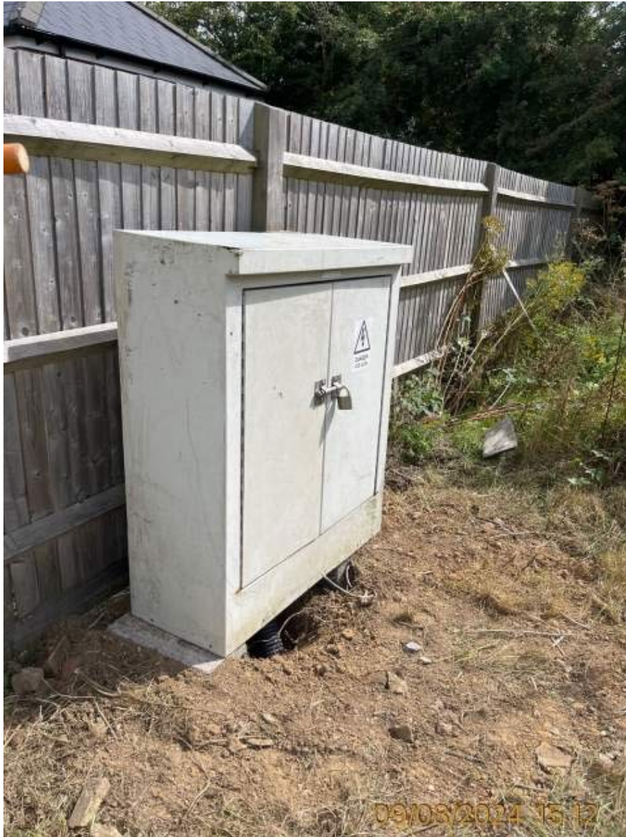
Plate 11 – A power substation at site entrance. Visible power lines going underground.
