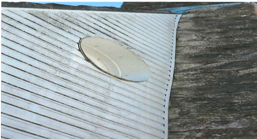
Picture 3: Showing the gaps around the UPVC cladding and the lead flashing.
