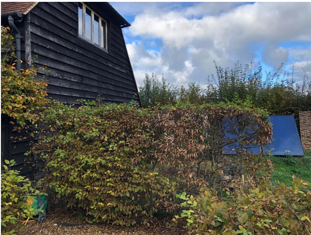
PHOTO 2: VIEW LOOKING NORTH HORNBEAM HEDGE SCREENING HEAT PUMPS, SOLAR PANELS BEYOND
