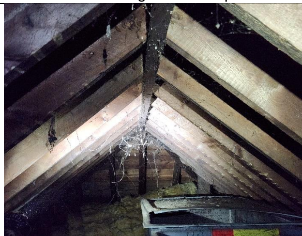
Photograph 17: Cobwebbed roof void within the Main House.
