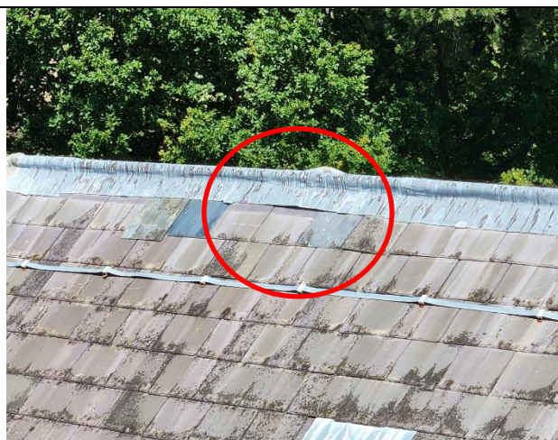
Photograph 16: Lifted lead flashing on the Main House creating a crevice space.
