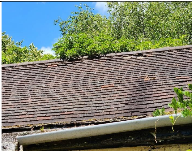
Photograph 31: Gaps in the southern roof pitch.
