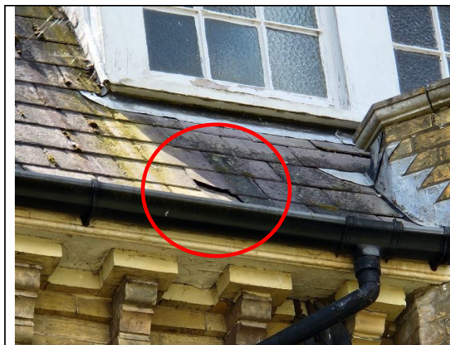
Photograph 15: Broken roof tile on the Main House creating a crevice space.
