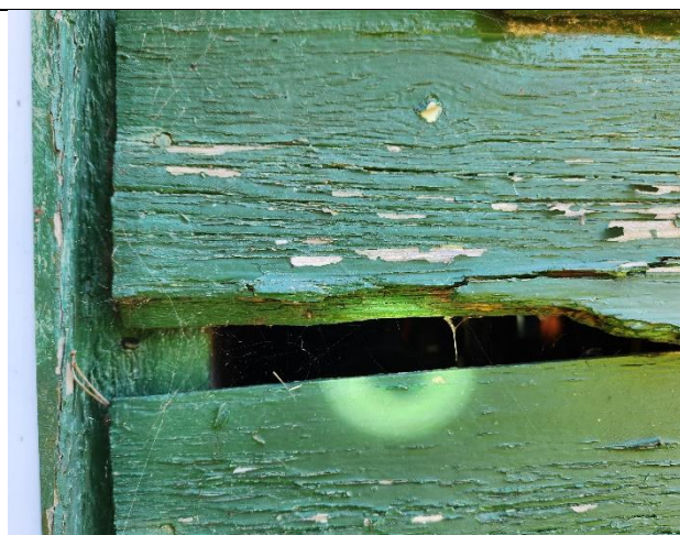
Photograph 26: Gap into the Barn through a damaged wall.
