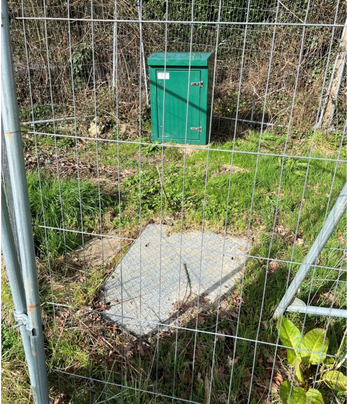
Pumping station and control kiosk
