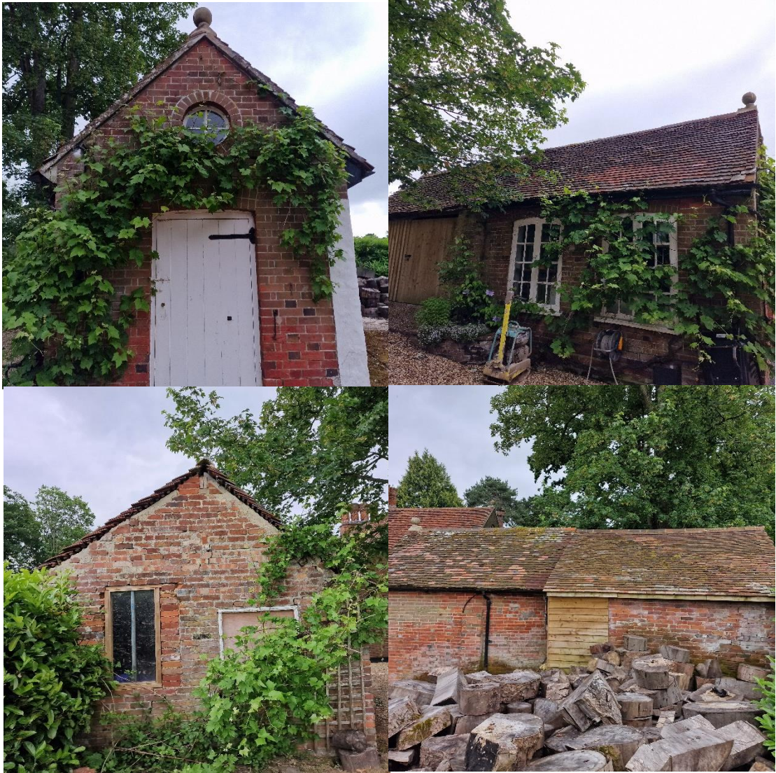
Photo 1: The four aspects of the outbuilding showing lifted tiles and gaps along the roof line
