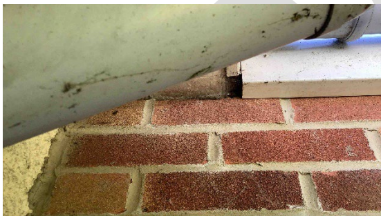
Photograph 5. B1 - fascia gap west aspect
