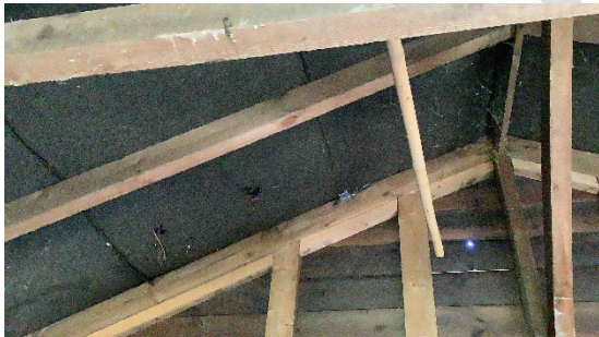
Photograph 13. Holes in roof lining of B2
