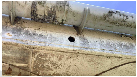
Photograph 4. B1 - hole in fascia north aspect
