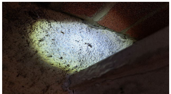
Photograph 8. B1 – Bat droppings below soffit hole in photo 7.
