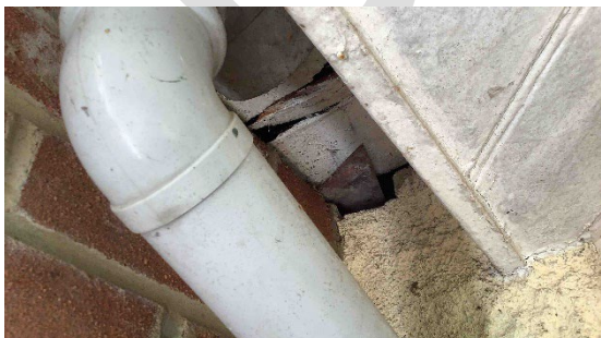
Photograph 7. B1 – south aspect soffit hole (bat droppings below)
