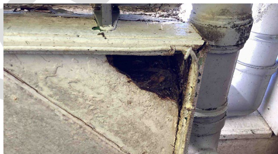
Photograph 6. B1 – soffit hole south aspect
