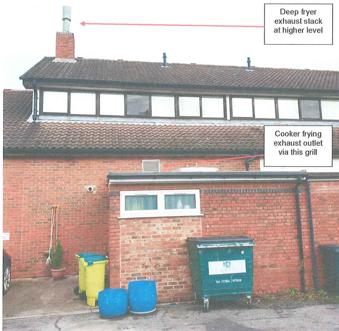
FIGURE 2 The extraction outlet grill at rear of Chunky at Pilgrims Close
