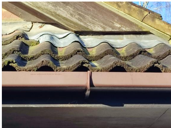
Photograph 6: Gaps under the lead flashing and roman tiles on the mono-pitch roof on the eastern elevation of the building.
