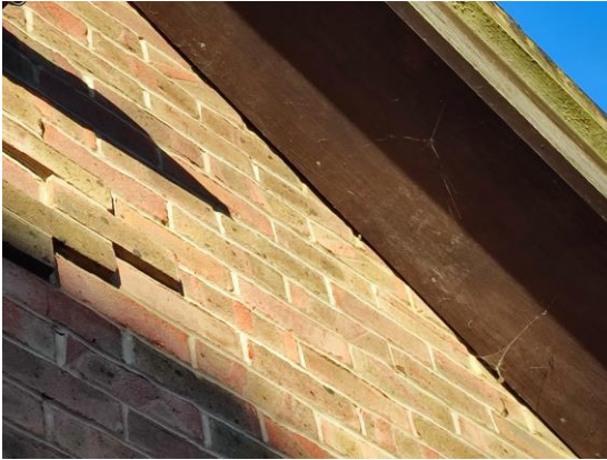
Photograph 7: Gaps where the soffit meets the wall on the eastern elevation of the building.
