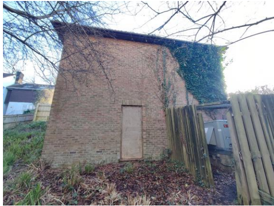
Photograph 10: Western elevation of the building. Ivy covers most of the south-west corner of the building.
