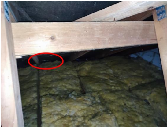
Photograph 15: Light can be seen entering the roof void from the eaves on the northern side of the roof void.
