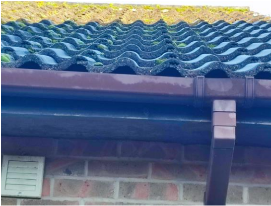
Photograph 9: Gaps under the ends of the roman tiles on the southern elevation of the building.
