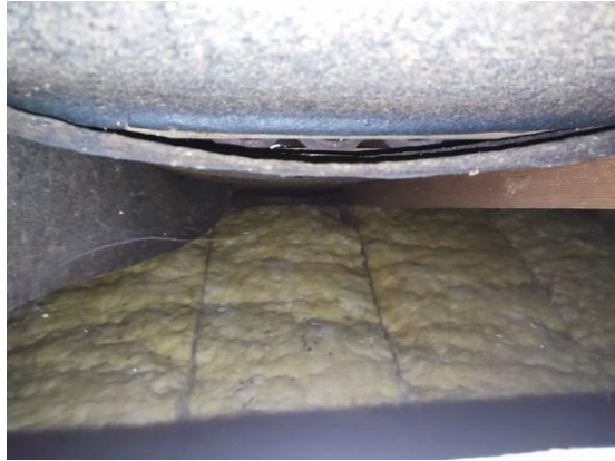
Photograph 14: Sagging bitumen felt and an exposed roof tile with gaps providing a potential access point for bats into the roof void.
