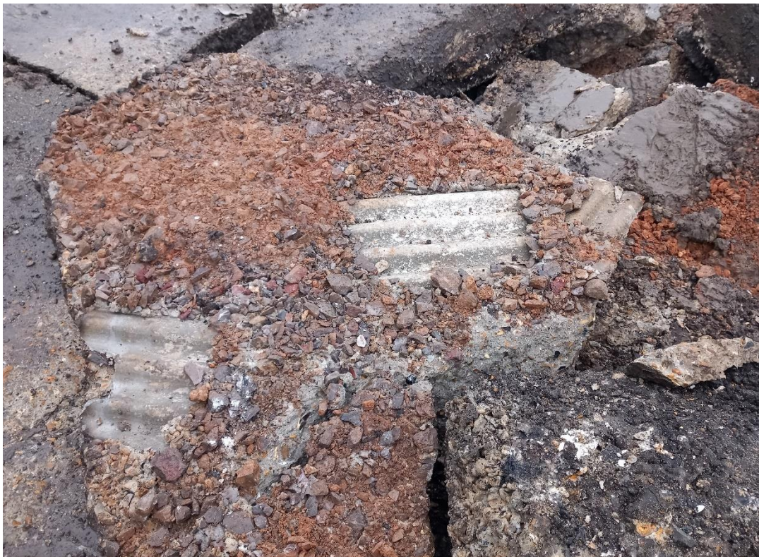
Plate 10: Site Visit 19/12/22 – Observed two sheets of corrugated suspected ACM roof tiles
