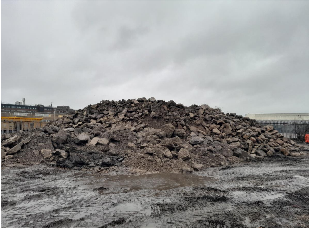
Plate 21: Site Visit 09/01/23 – Broken out concrete stockpile
