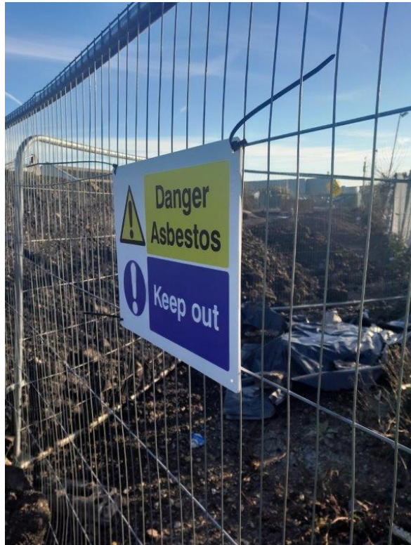
Plate 25: Site Visit 23/01/23 – Segregated and Covered Suspected Bound Asbestos encountered (i.e. identified corrugated material bound to base of exposed concrete slab – see Plate 10)
