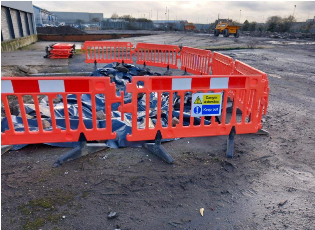
Plate 16: Site Visit 21/12/22 – Covered and securely fenced suspected asbestos areas
