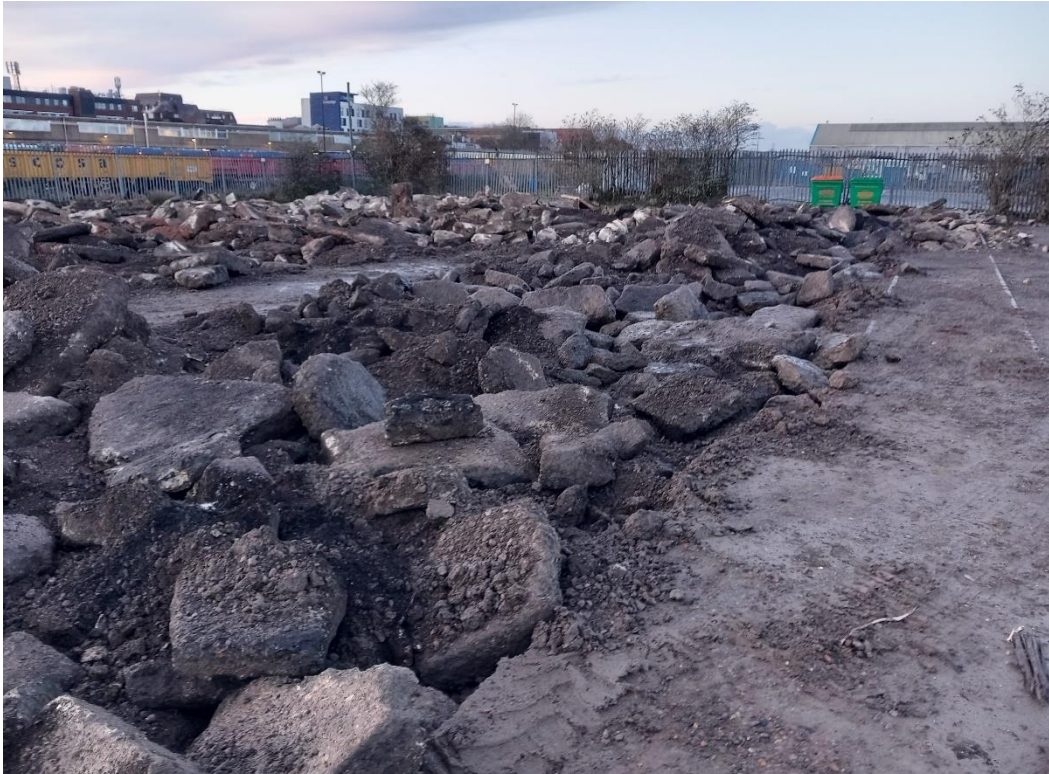
Plate 17: Site Visit 21/12/22 – General broken out material in west of the site
