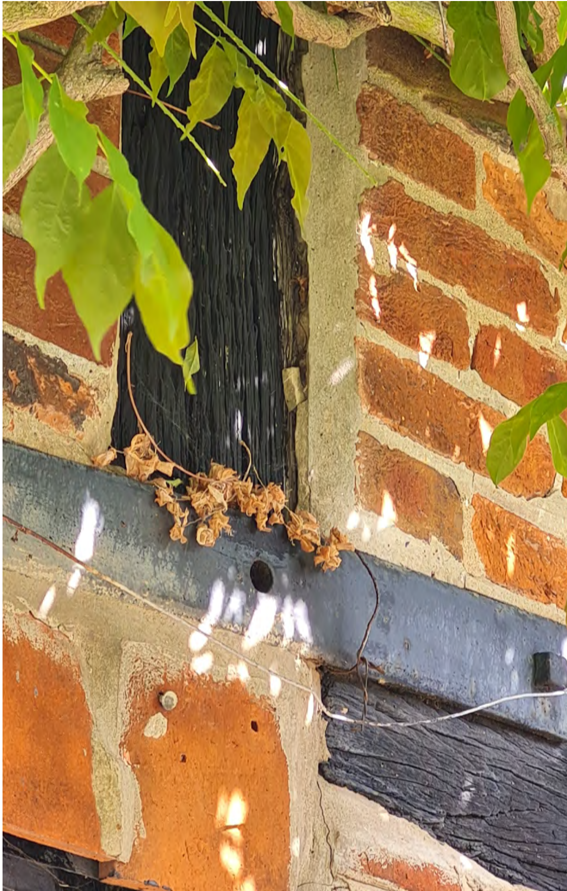
Figure 14; Close-up view of the junction of a masonry panel below the dormer window at its junction with the adjacent post to the timber frame. Note the outward movement of the panel, even beyond that from the cementitious shoulder which is itself relatively modern. The gapping gets worse as the panel leans outward toward the top, but this is obscured by the Wisteria.
