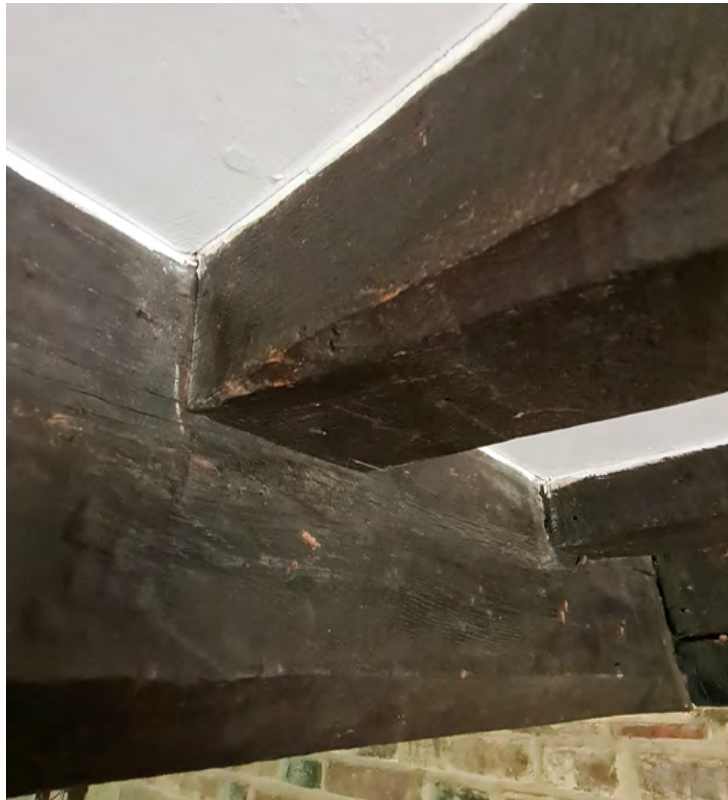
Figure 35; Image of the run out stop to a typical floor joist in the Living Room where it meets the primary beam. Other joists to this room have no chamfer at all, and hence no stops.
