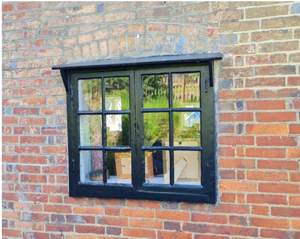
Figure 30; View of the slightly face-planted window beneath the brick arch.
