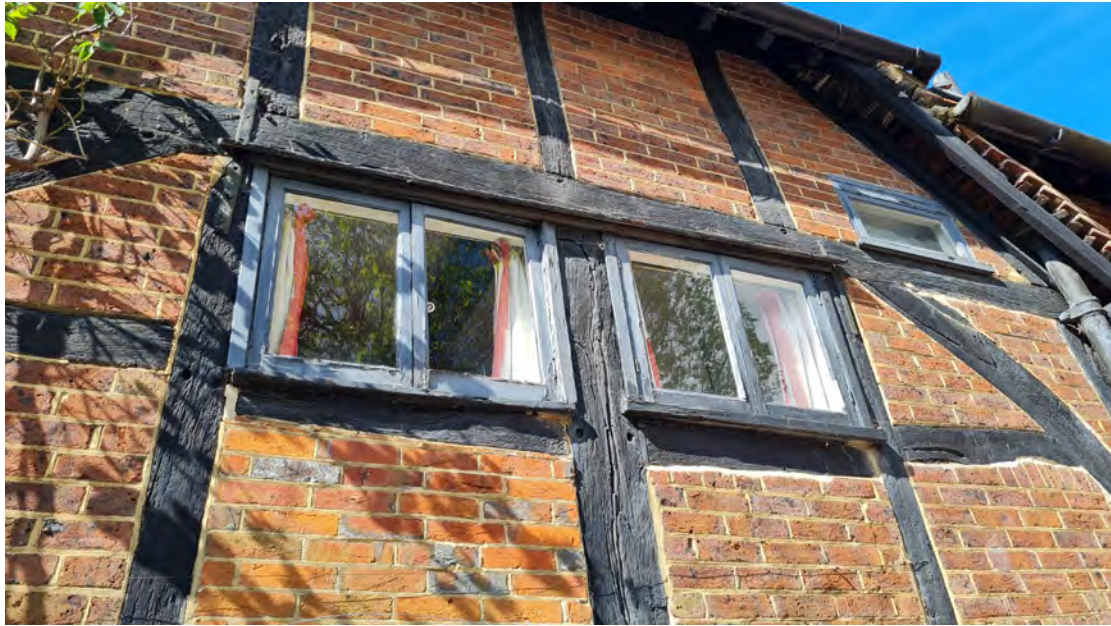
Figure 25; The very poor quality and poorly detailed modern first-floor bedroom windows to the North-East elevation, with the bathroom window up and to the right. Note the one more traditionally coloured brick panel above the girt is visible below the left-hand window.
