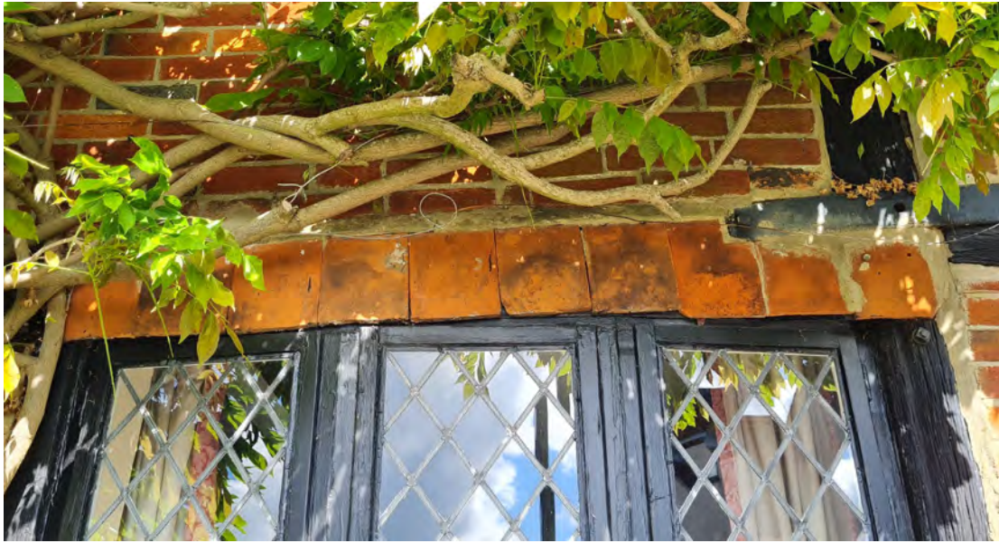
Figure 12; Close-up view of a section of tile covering above the window head. Note also the poor quality of the modern bow window.
