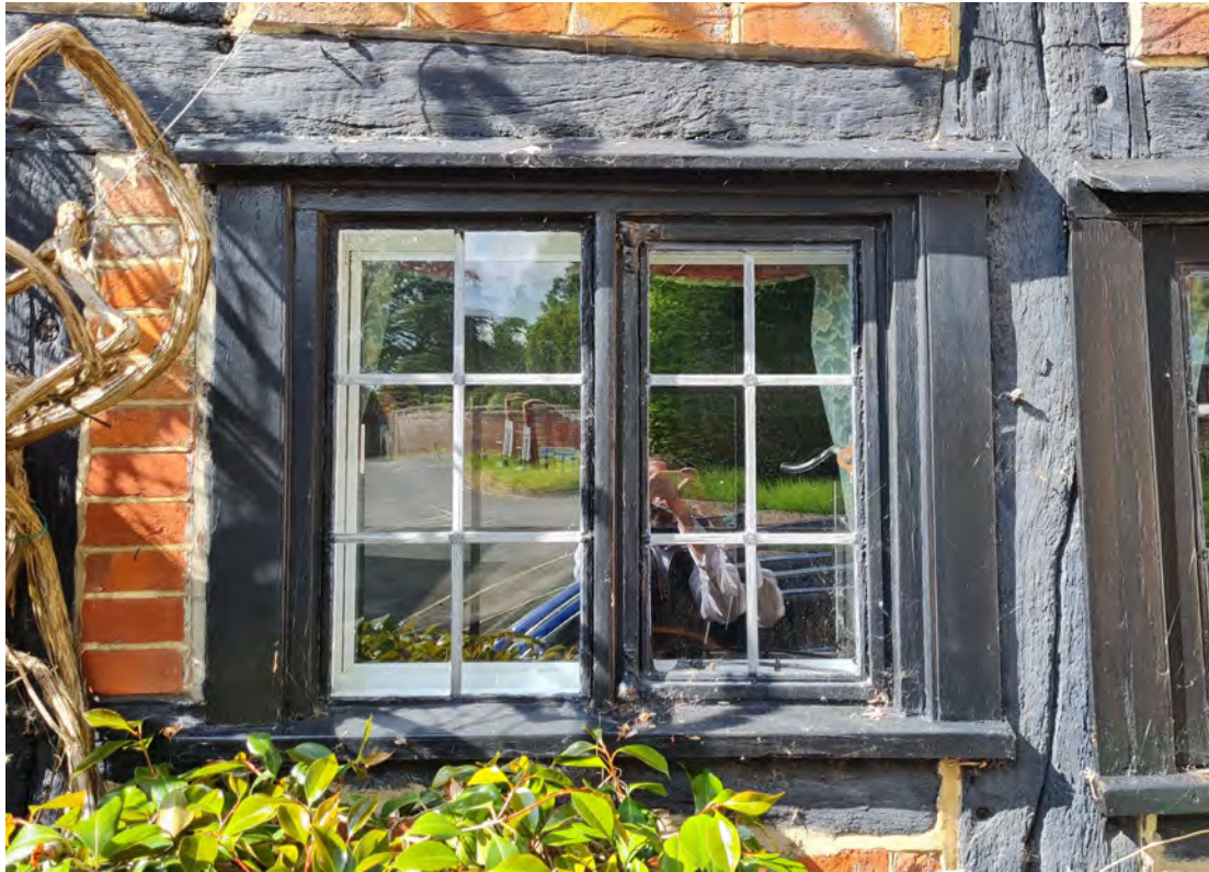
Figure 23; The left-hand of the ground floor windows to the North-East elevation, showing the steel casement, and basic rather poor-quality nature of the joinery.
