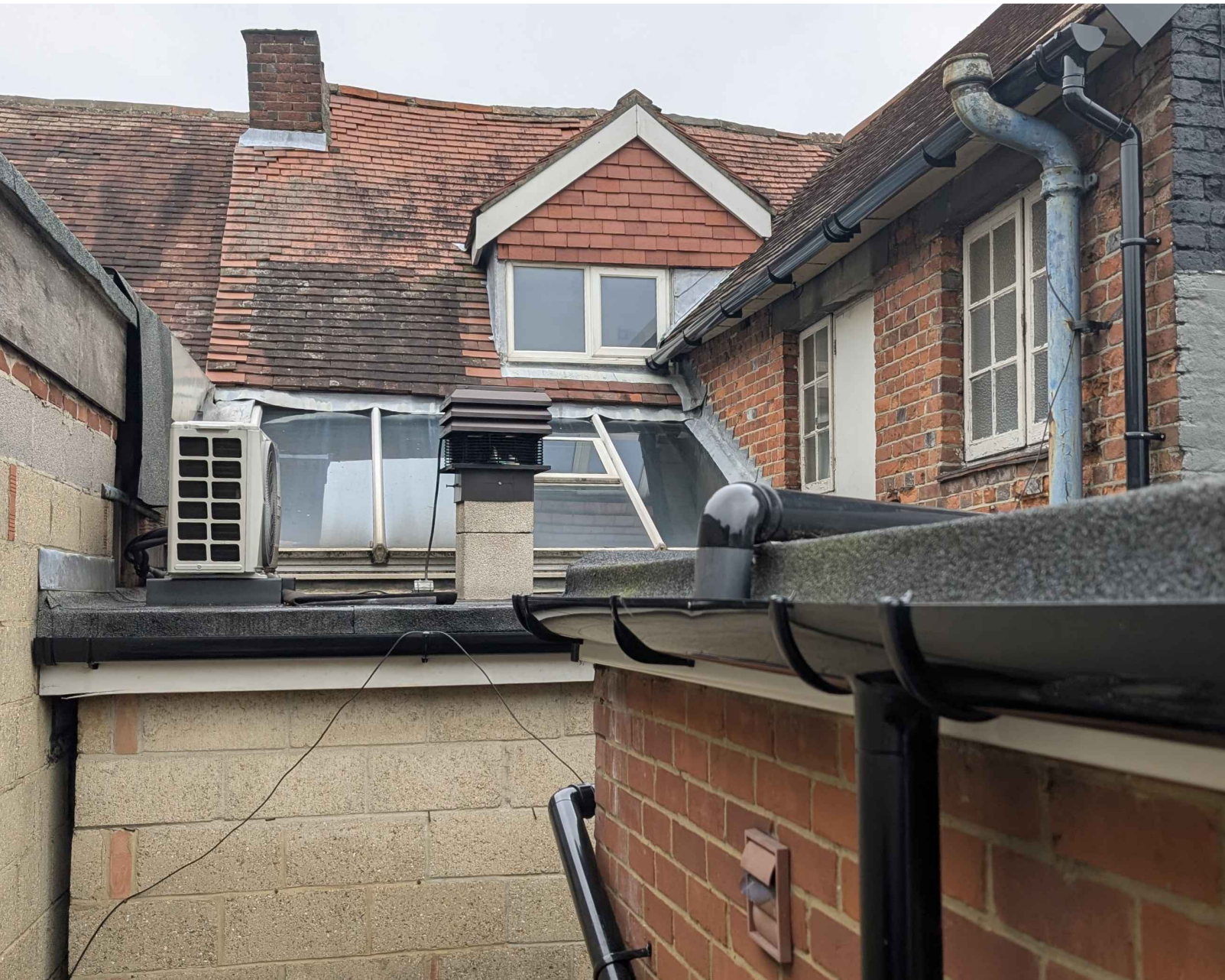
Photograph of extractor fan installed on site
