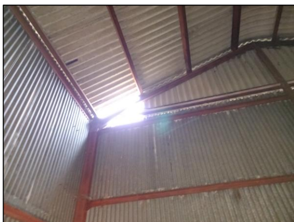
Photo 5 Gaps in corrugated panelling
