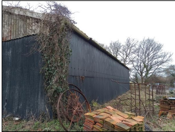
Photo 7 Eastern elevation – guttering at eaves
